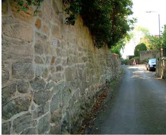
Above left - tall random rubble walls of local gritstone along Salsbury Lane
