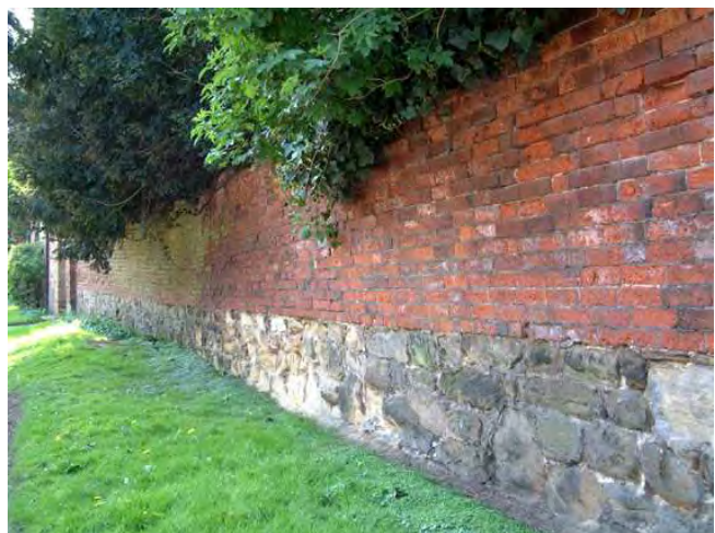
Below right - tall walls of red brick with an earlier stone wall used for footings at Chantry House, Church Street
