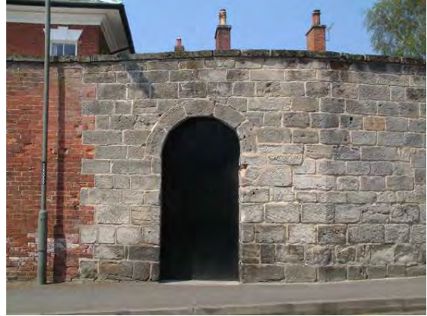
Above right - tall coursed gritstone walls at The Grange, Pack Horse Road (over 3 metres high)
