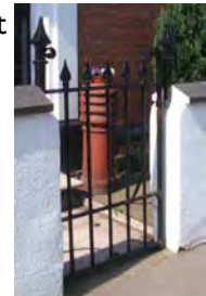
Below left - hand-forged railings in steel, fabricated in modern times to replicate the original wrought iron spear-headed pattern (15 Potter Street).
