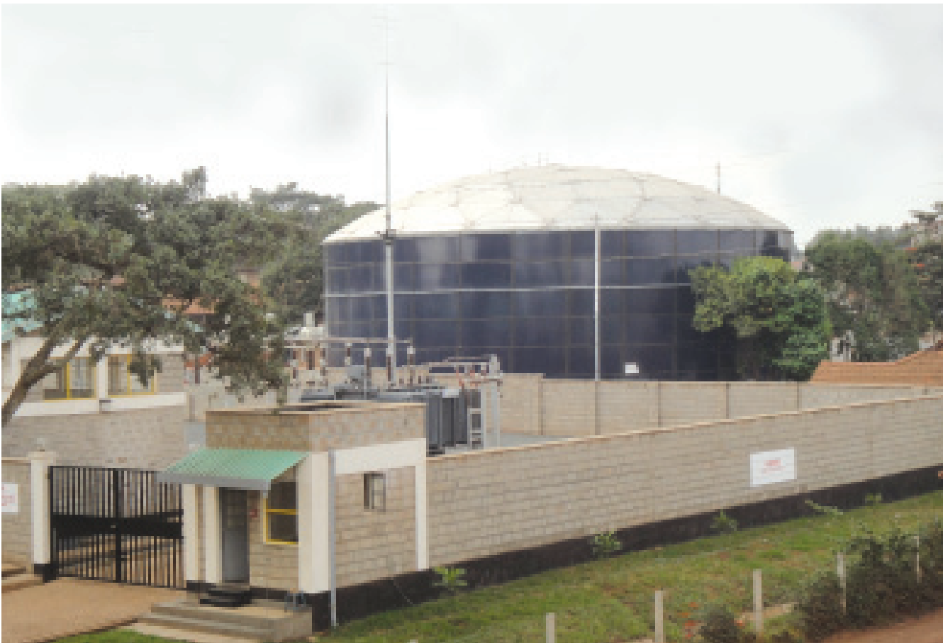
Foreground: The 66kv power supply line. Background: The new 4000m 3 water storage tank
