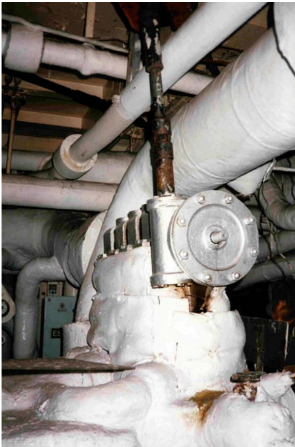
HMS Plymouth Starboard Turbine Nozzle Valve Gear
