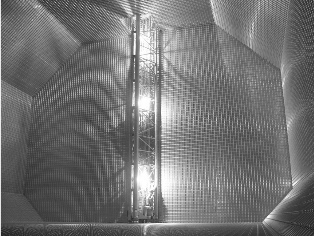
Figure 4-9: GTT Mark III - Courtesy GTT
