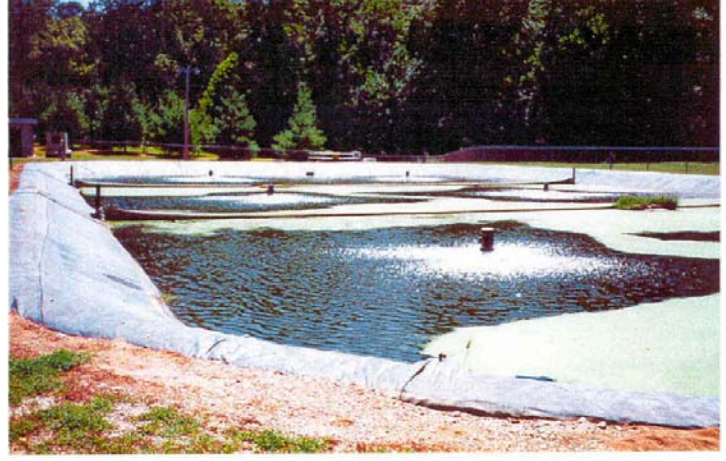
Three-cell sludge basin with chlorination facilities in far background
