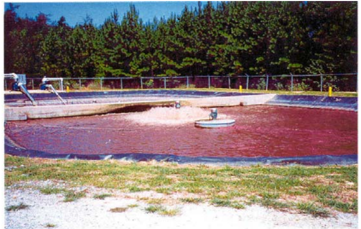
Closer view with decant and mixed-liquor recycle pumps in left background
