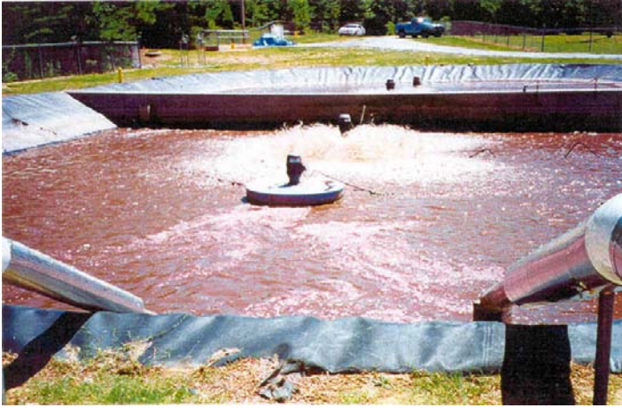
Second cell of reactor basin in foreground with headworks in far background
