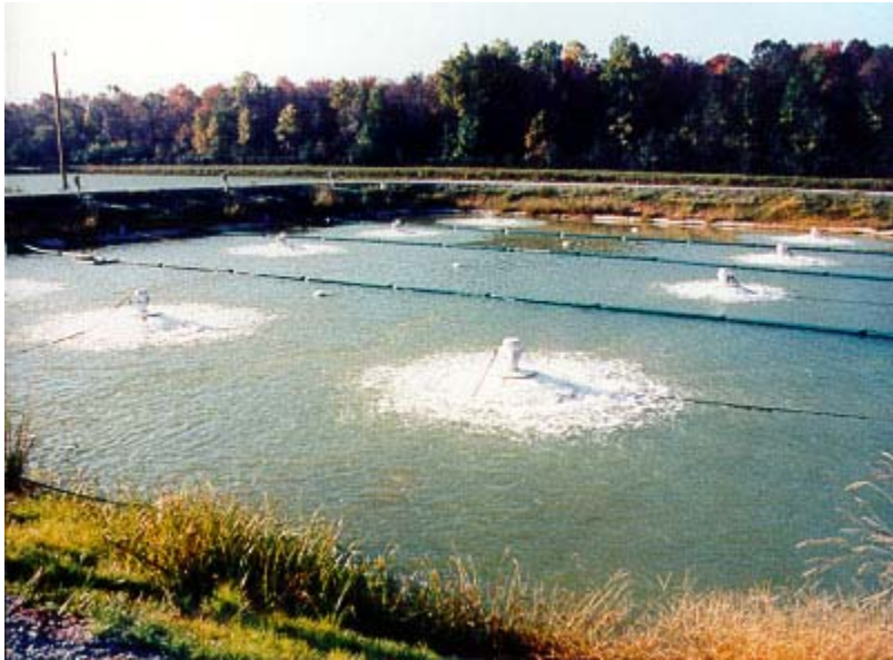
Figure 3. Photograph of a DPMC aerated lagoon system
