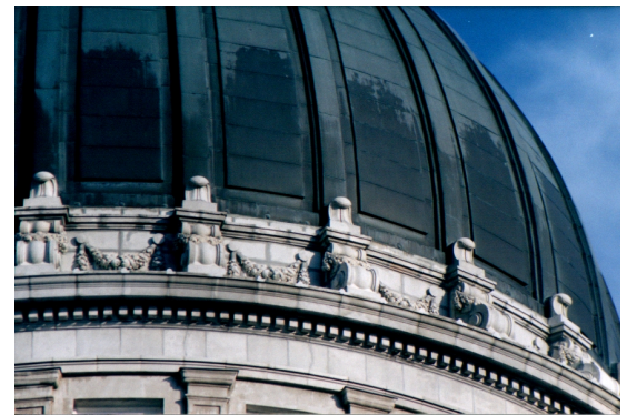
SHEET COPPER PATINIZING (OXIDIZING) ON THE ROOF OF THE DOME
