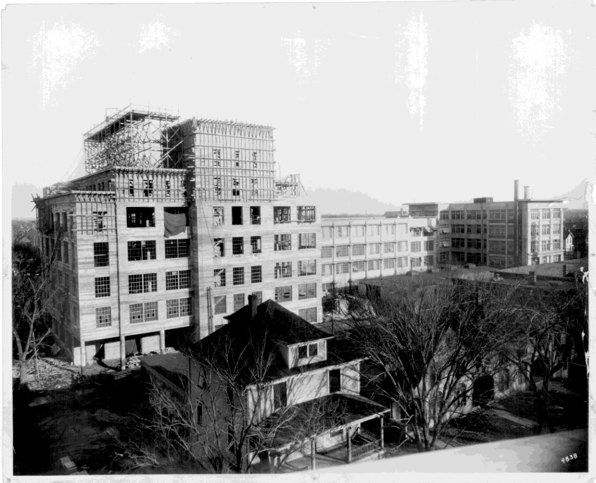
Figure 4: Historic image, Buzza Company Building expansion and tower, under construction, ca. 1927. View looking southeast towards west elevation. (Hennepin County Library, Minneapolis)
