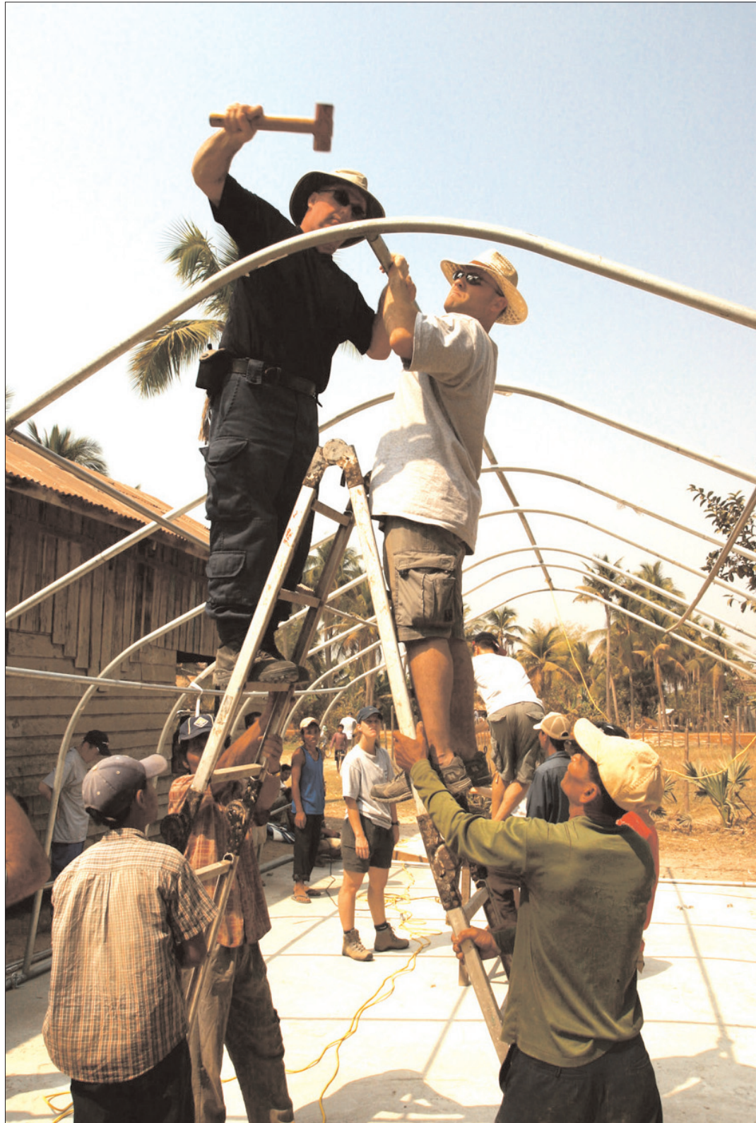
Sgt. Don Ryan and Const. Dave Phillips assemble a structure with help from Cambodian workers
