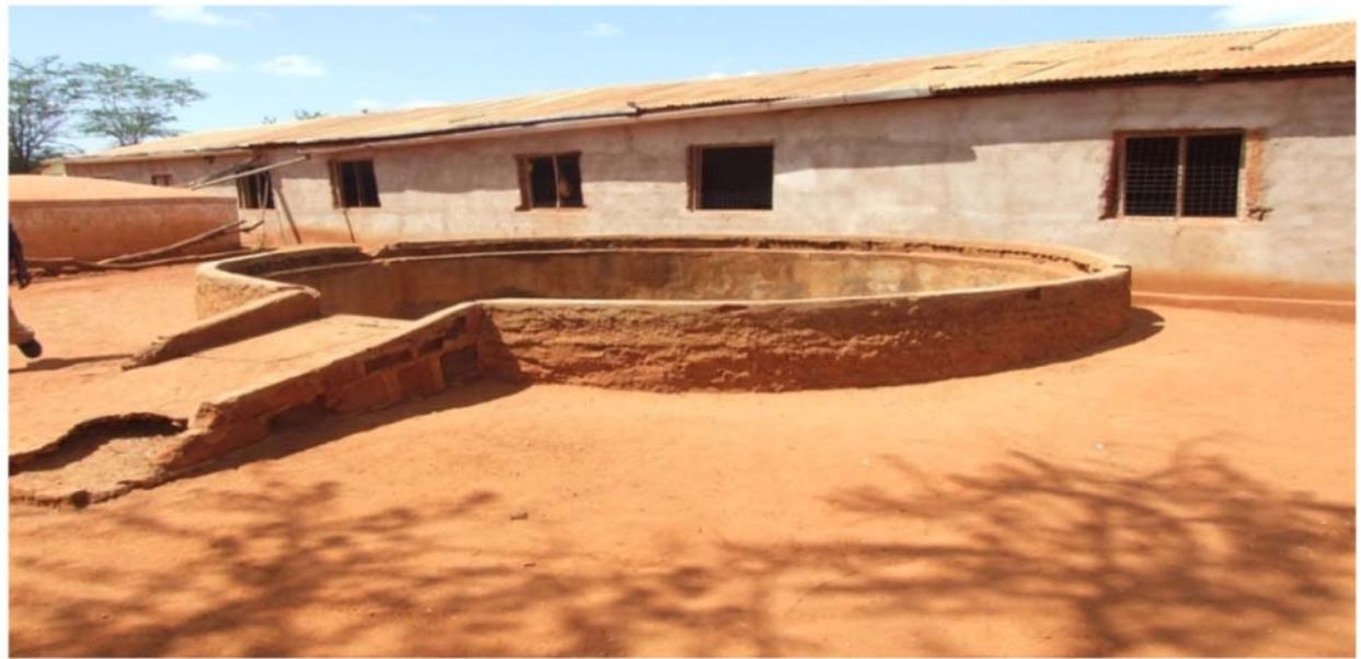
The tank at Ekani primary: old one fell apart and far left the new one.
