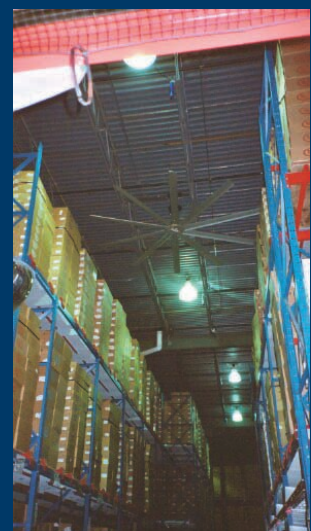
Figure 3 – large ceiling fan over warehouse storage racks
