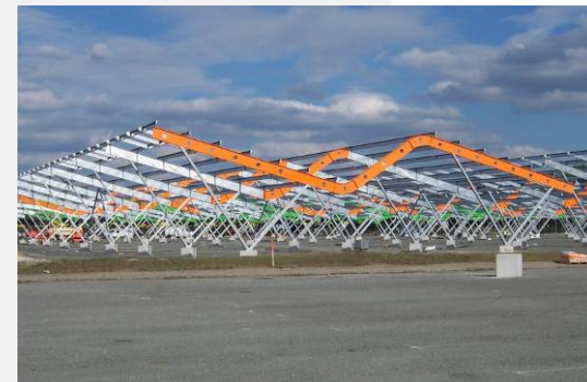
Photovoltaic panels supports - Vilquin
