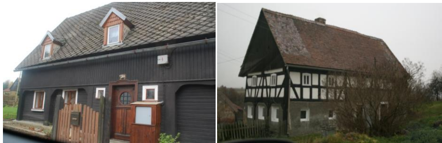
Fig. 41. Examples of various traditional types of roof cover for umgebinde houses. From the left: slates and ceramic tiles [Author's photographs].
