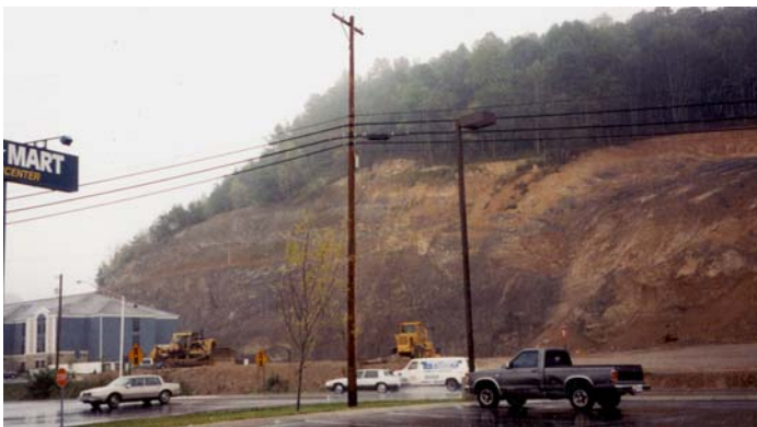
Figure 16. Collapsed terrace block along modified crater rim, Middlesboro, Kentucky at stop 7.
