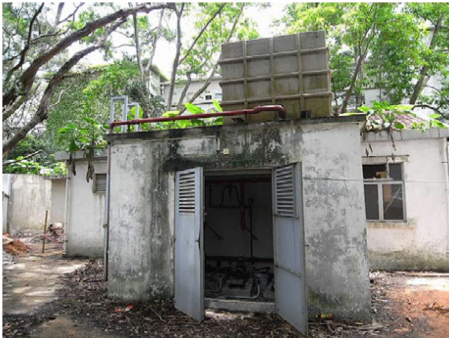
One of the two single storey buildings next to Duty Lawyers' Office accommodating mechanical equipment and water tank
