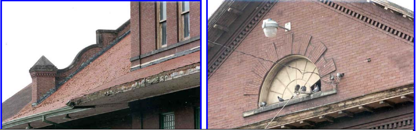
BEFORE: A deteriorated roof, broken windows and tons of pigeon residue had to be removed.
