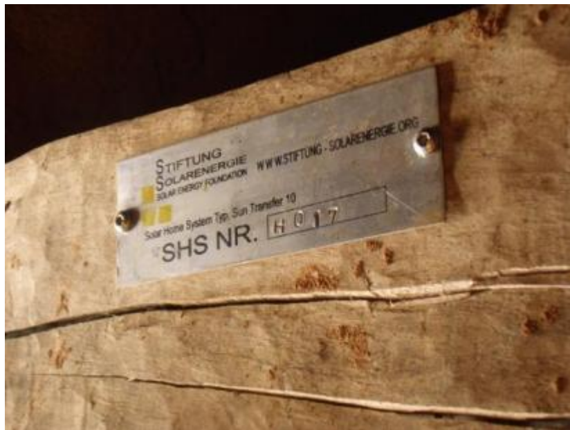
Picture 11: The solar households are numbered and recorded.
