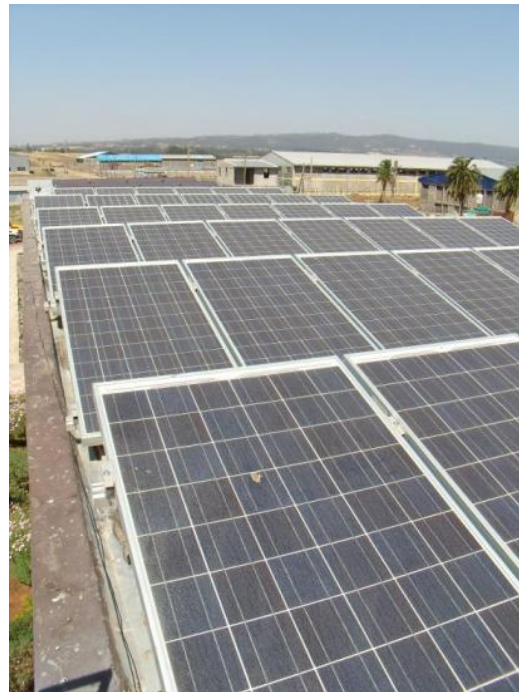
Picture 6: Solar modules on the roof of the school building, providing electricity for Solar Valley (at present stand alone).
