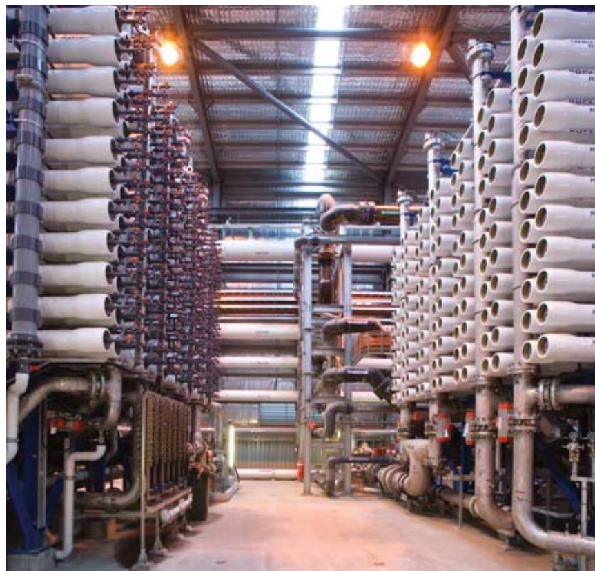
Gibson Island Advanced Water Treatment Plant
