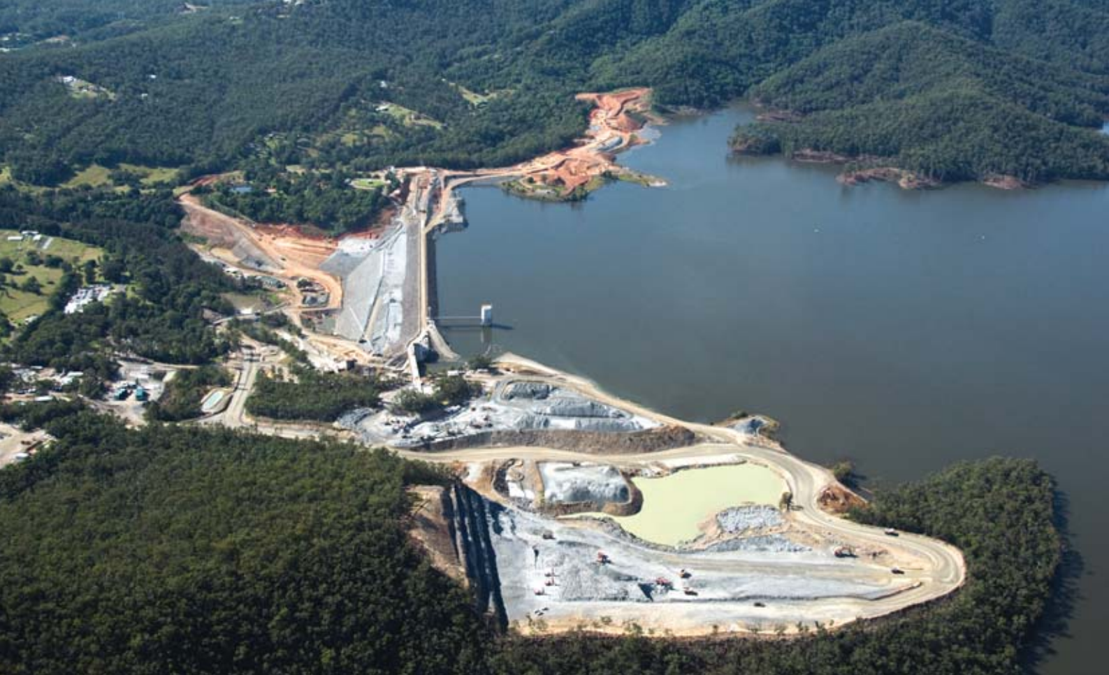
The Hinze Dam Stage 3 Project will increase water supply from the dam to 225 million litres a day.
