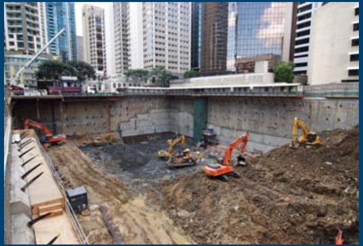
Vision Mary St – Brisbane Diaphragm and Secant Pile Retaining Wall for bulk excavation depth 22 metre
