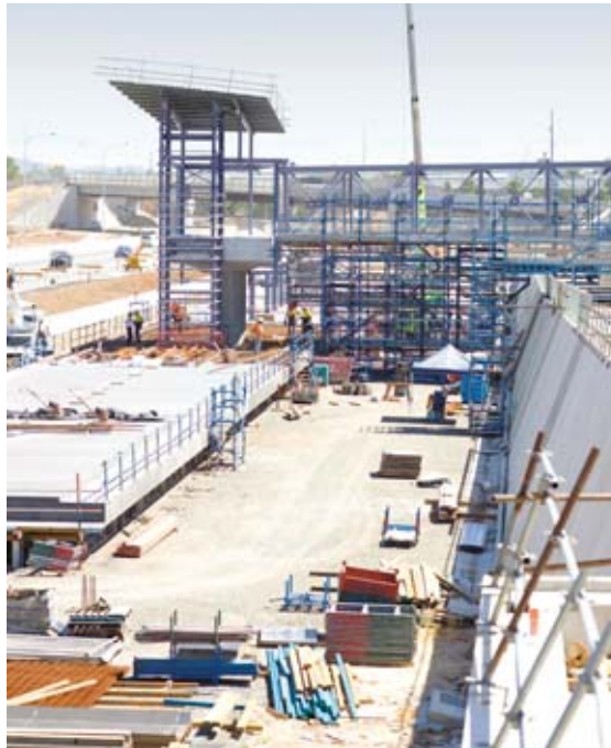
Richlands Station taking shape in January 2010, part of work on the Darra to Springfield Transport Corridor
