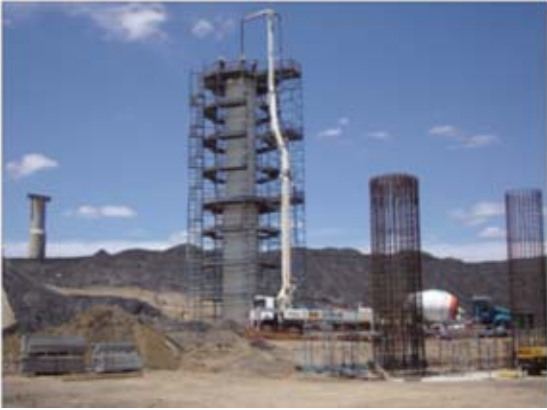
Stockpile Conveyor Tower.
