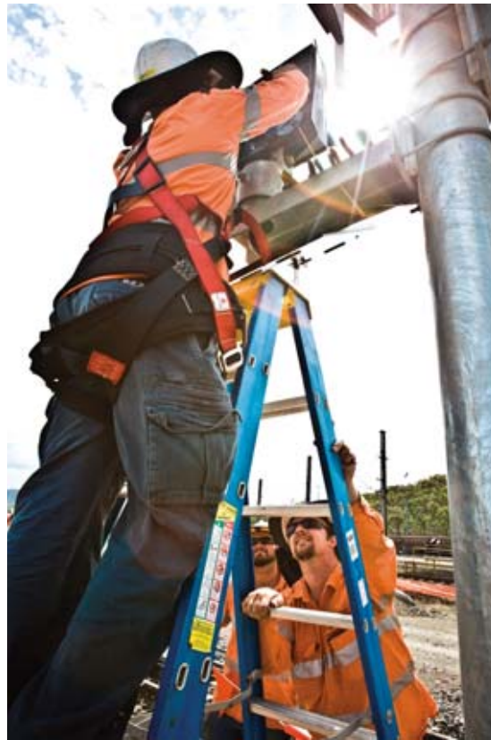
Workers on the Jilalan upgrade: ZERO Harm is QR Network's core value.
