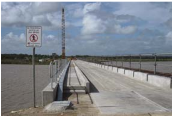
Work on the now completed St Lawrence Creek Bridge – improving reliability of rail services on the North Coast Line.
