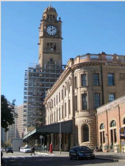
Scaffolding of Central Station Clock Tower enclosed inside polyethylene to ensure maximum safety protection of the public.
