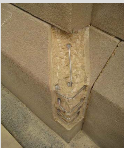
Stainless steel reinforcements typical of synthetic repair patches.
