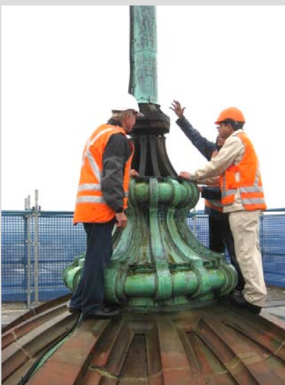
The reconstructed flagpole being inspected (above) and being craned into place (right).
