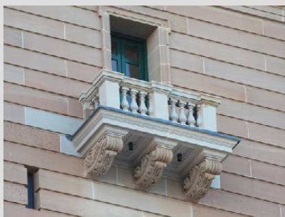
The Clock Tower's Juliet balcony before and after restoration. Light coloured stones are those that have been replaced or indented, including the 4 ton floor slab stones.
