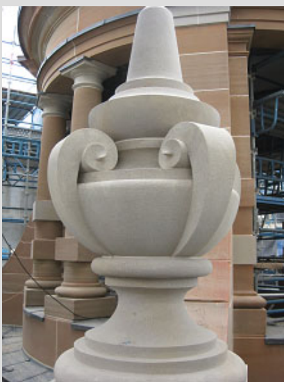
New stone urns stored on site (right) ready to be hauled via pulley up to the Clock Tower, and the new urns reconstructed (above).
