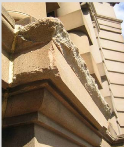
Stone defects to cornices of Clock Tower.
