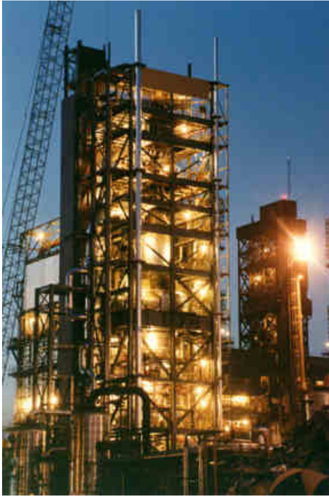
Hylsa 4M plant using reformerless HYL III technology with HYTEMP Pneumatic Transport System tied to the EAF minimill.
