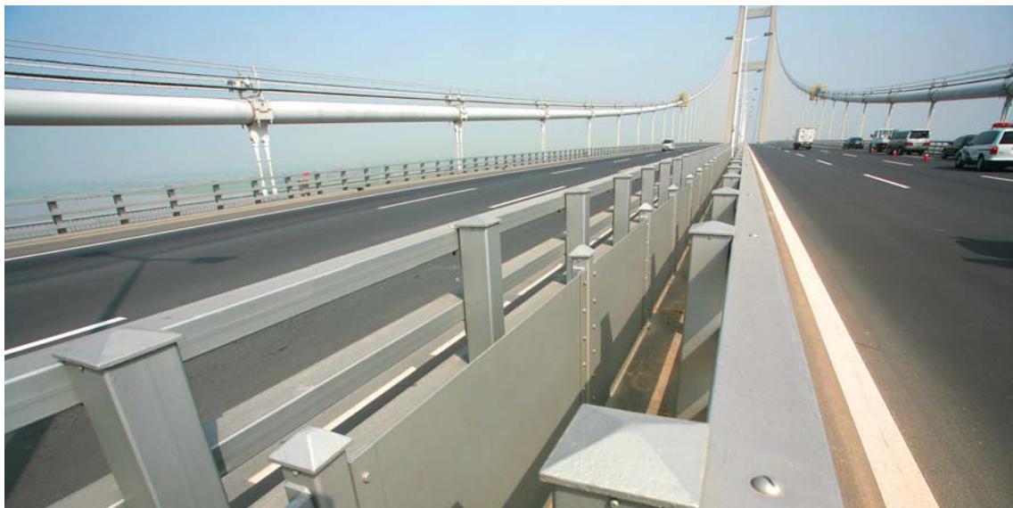
Figure 4: Central stabilizer mounted on the Jiangsu Runyang South Bridge
