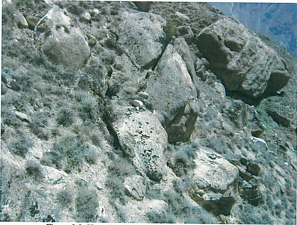
Figure 3.2: Huge boulders loosely lying on the baskslope
