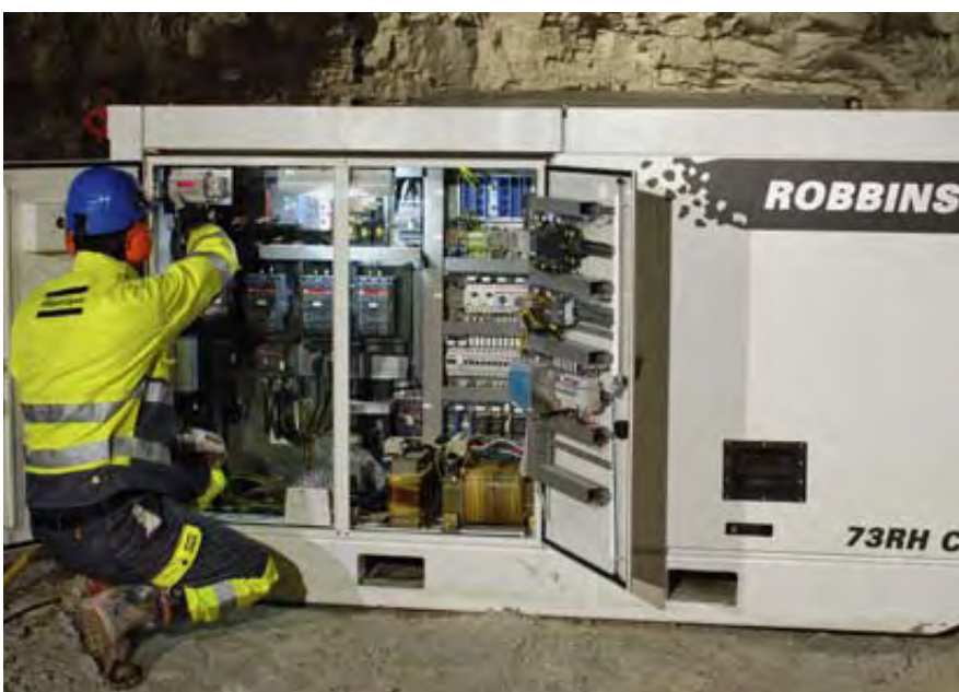
Figure 6: Electrical power unit.
