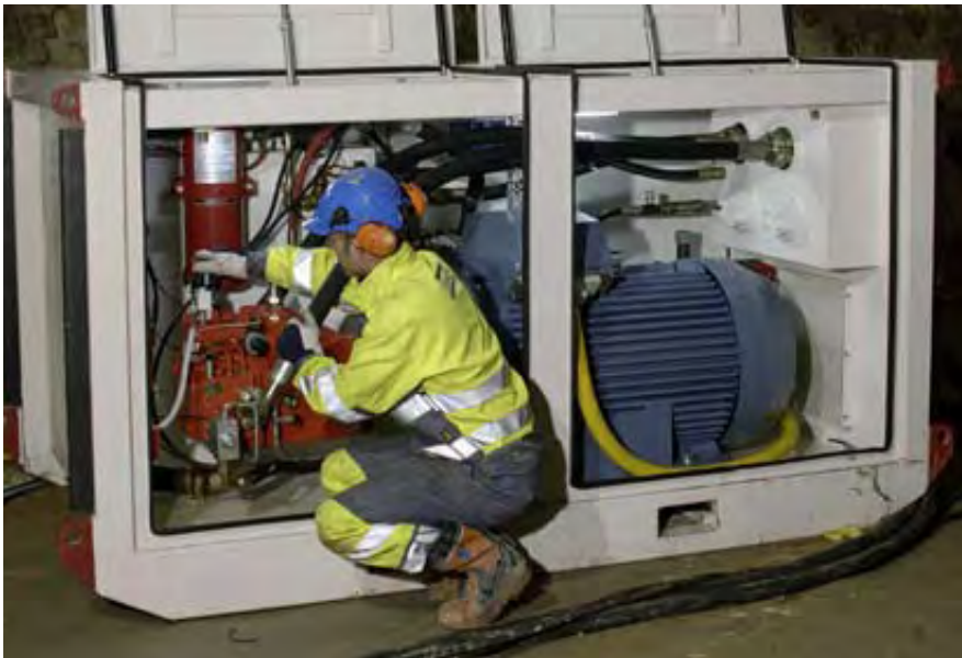
Figure 5: Hydraulic power unit.
