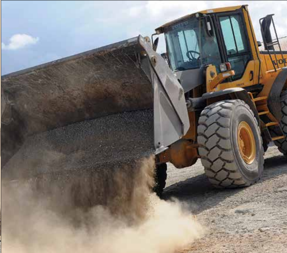
Air Force Staff Sgt. Marcos Diaz, heavy equipment operator assigned to the 474th Expeditionary Civil Engineering Squadron, dumps a large bucket of rocks to fill in ground at Camp America June 12.
