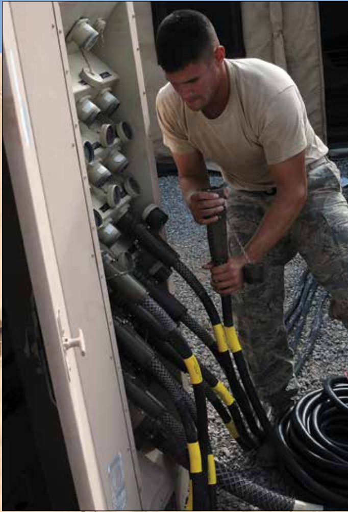
Senior Airman Alexis Vega, electrical systems technician, 474th Civil Engineering Squadron, plugs electrical cables into a power distribution center at the Joint Task Force Guantanamo's Camp America June 12.
