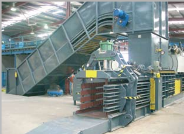
Baler installed at the Hobart MRF
