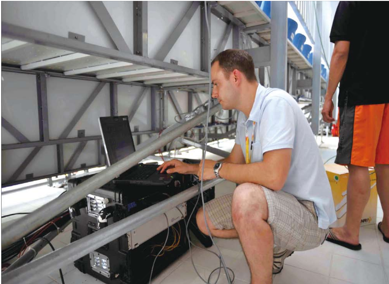
The WLAN devices installed in the photo work areas and the photo edition areas at the venues, which make high-speed data transmission possible
