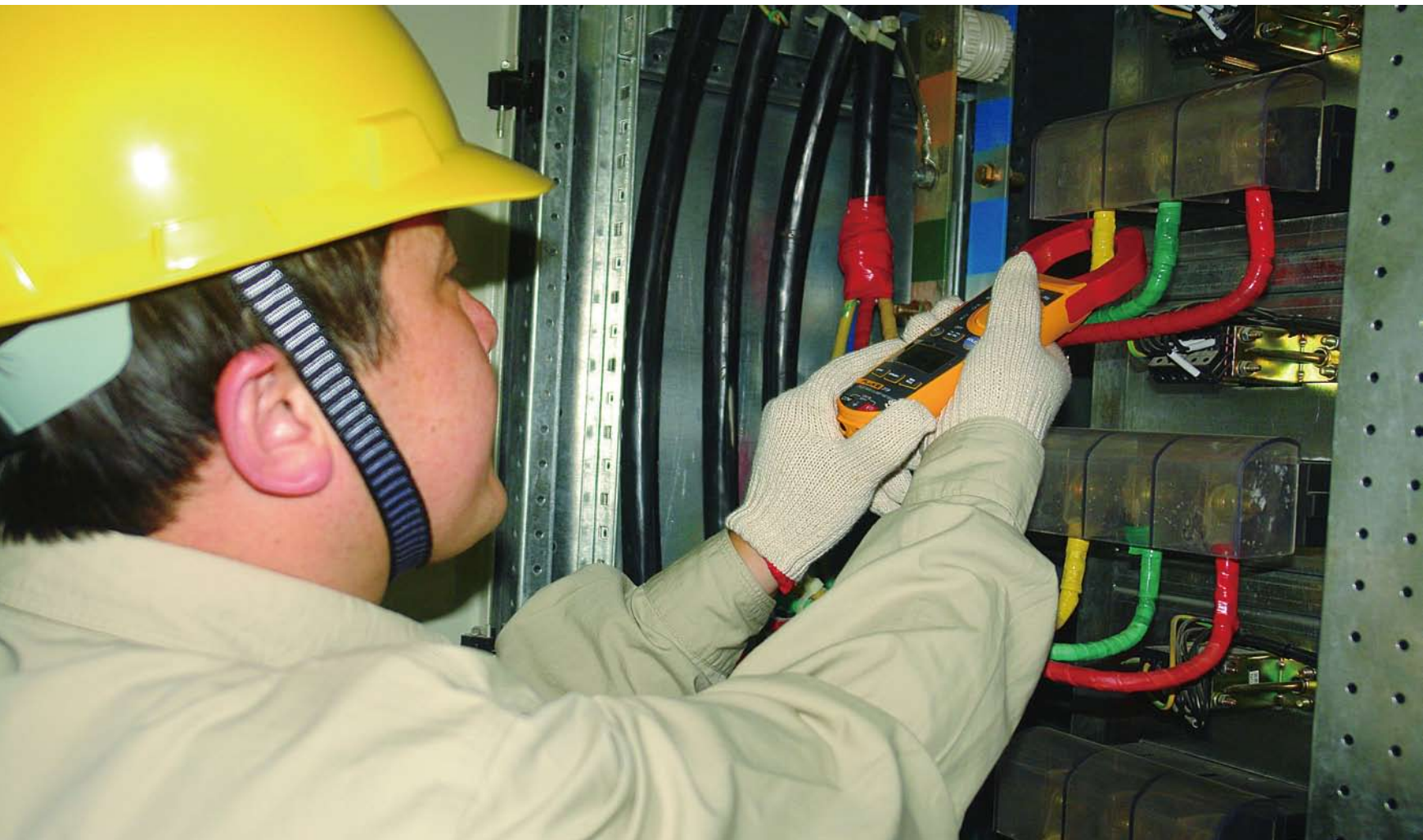
Staff from the State Grid test the power flow at an Olympic venue
