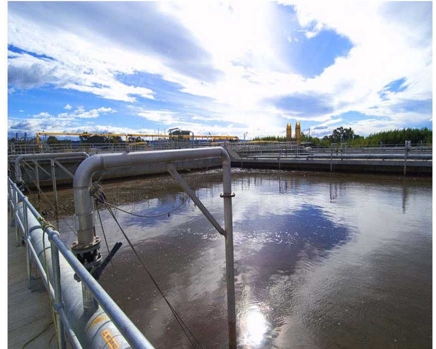
Sewage Treatment Plant, Penrith
