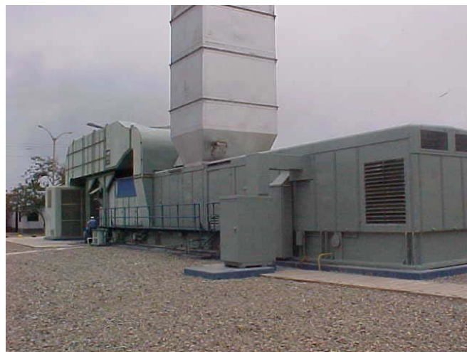
Turbina a gas
