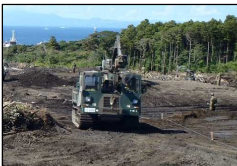
【Material carrier vehicle in action in the aftermath of a disaster on Izu Island】
