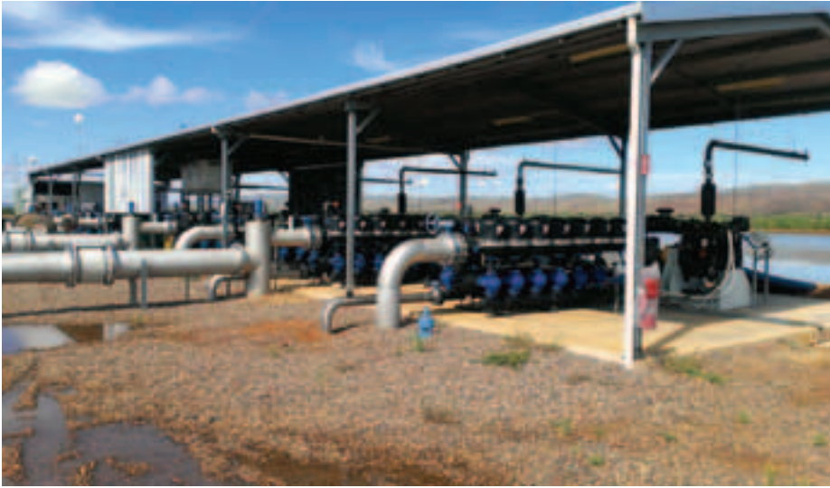
Above: One of the pump stations supplying water (2200 L/sec) to 1500 ha trees that are drip irrigated.
