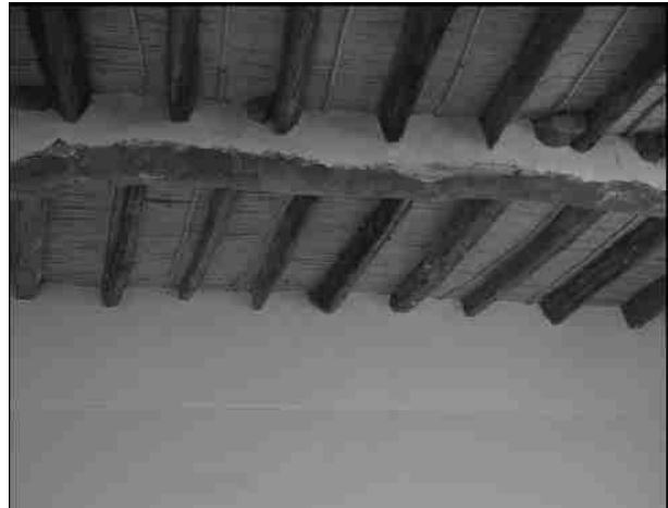
Figure 27: Typical roof of an Amazigh house: Asalas the bearer and his 'twin-brothers'.
