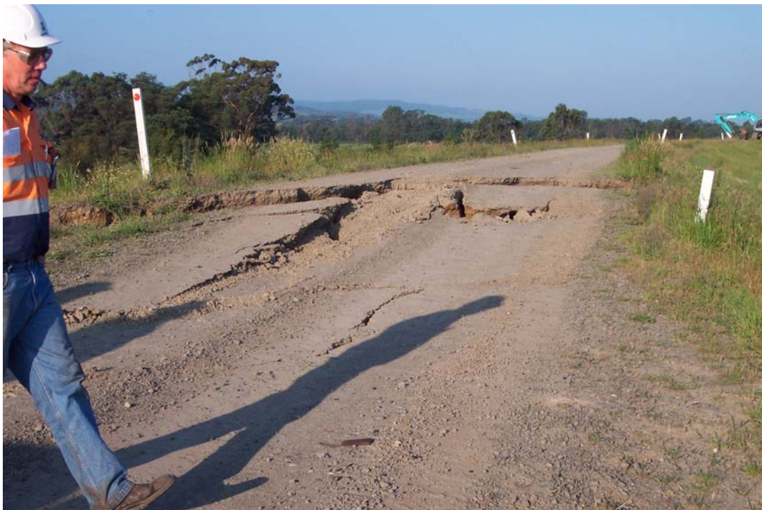
Figure 10: Cracks and subsidence across the Latrobe River Levee
