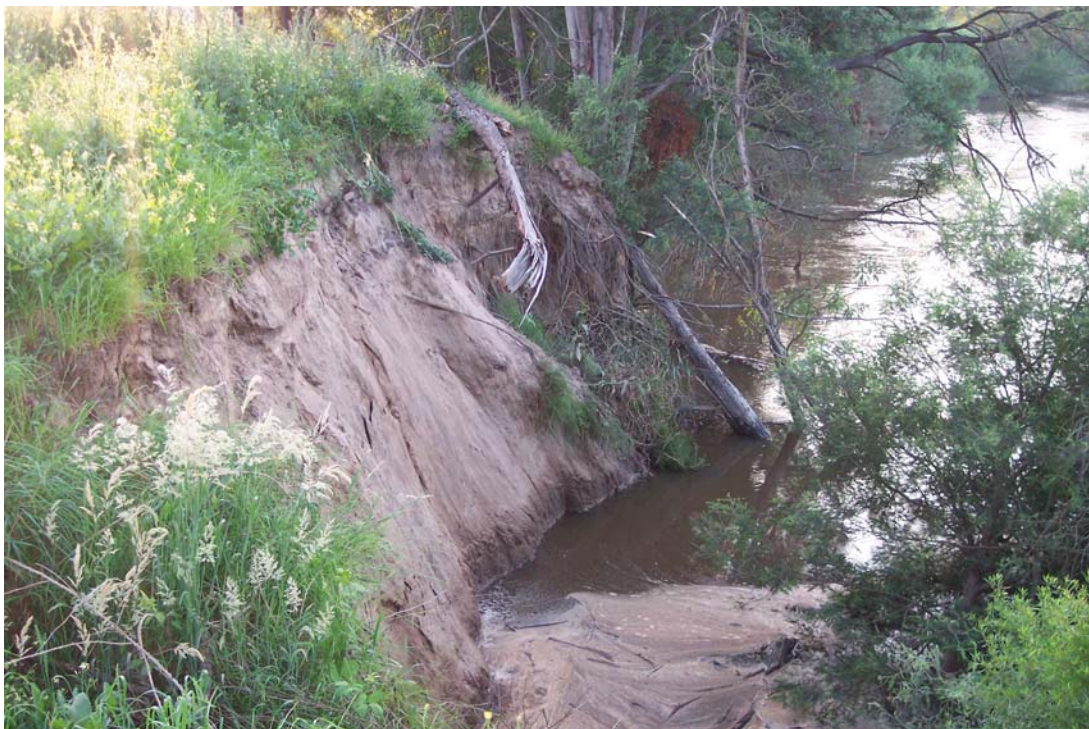
Figure 12: Crack in Latrobe River Floodplain and Latrobe River
