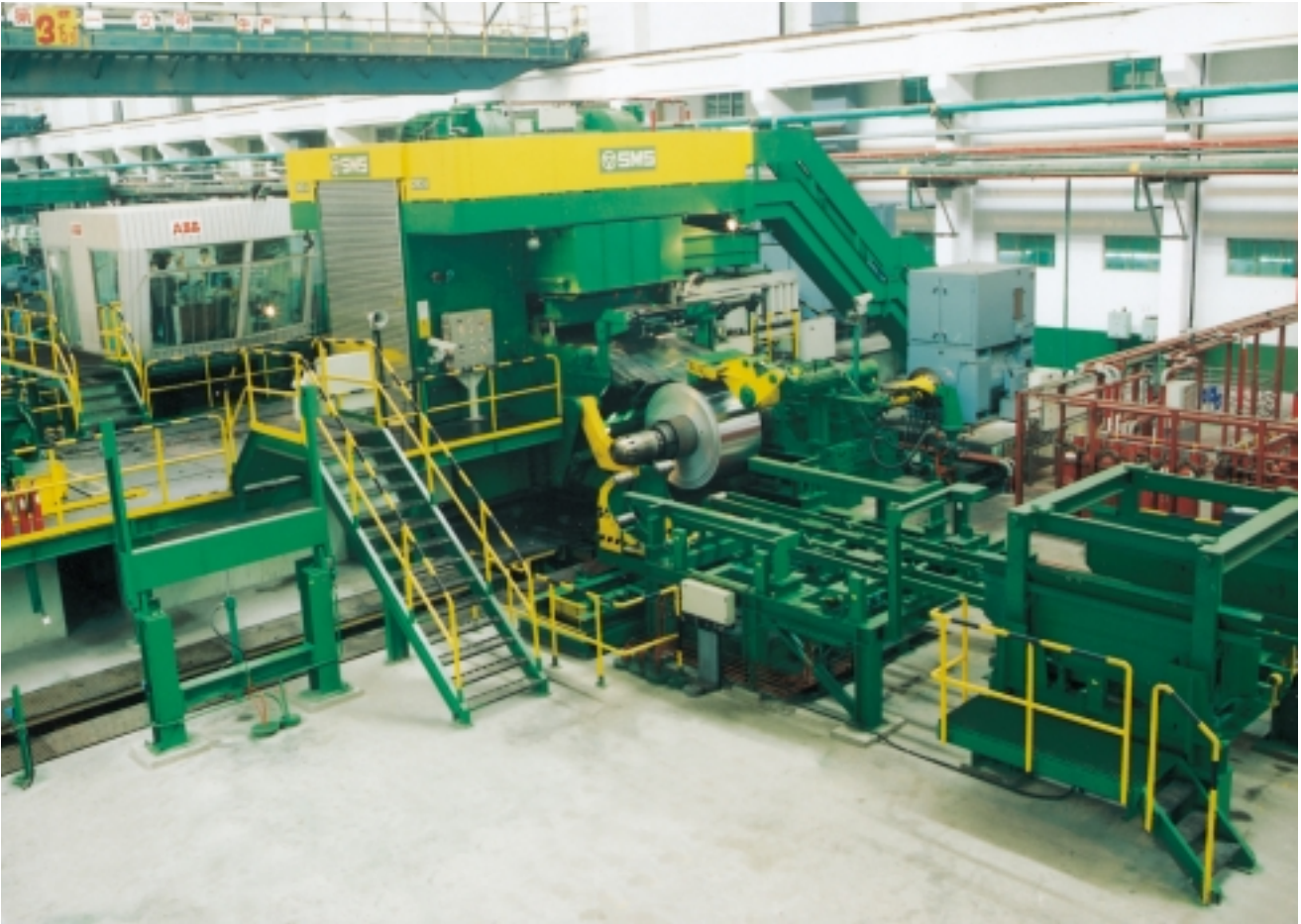
The new CVC four-high cold rolling stand of Southwest Aluminium in Chongqing-Xipeng, China. The stand was placed in operation by ABB in record time.
