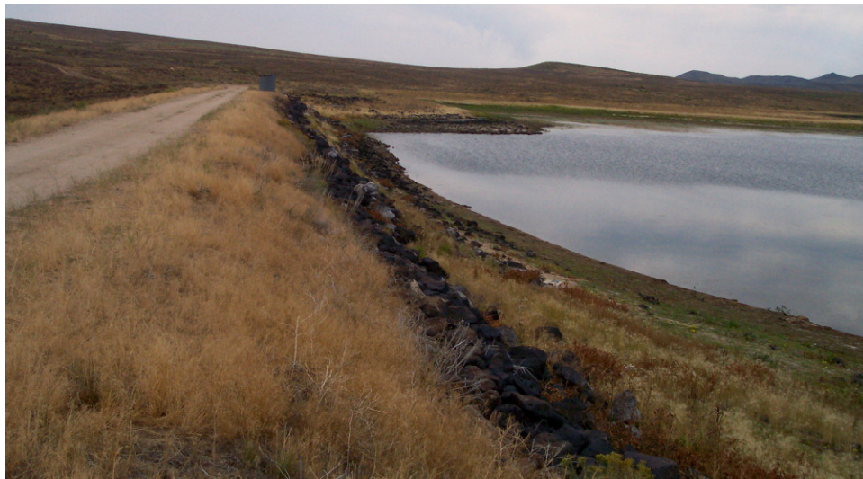
MORMON RESERVOIR (TWIN LAKES RESERVOIR) DAM SITE Picture taken summer of 1987, by Helen [retaken by Craig Dalton – August 2009]
