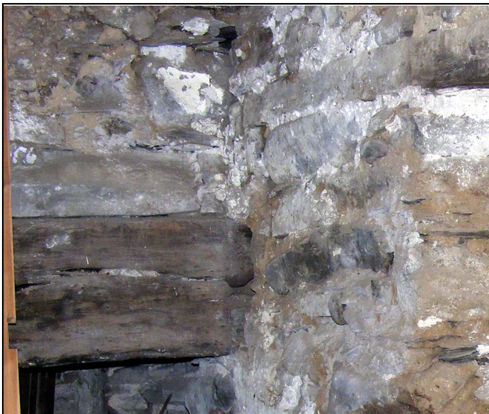
Figure 35 , The lintel of the fireplace (bottom left) with chimney wall above, hacked into the older south wall of the east range (E) to the right.
