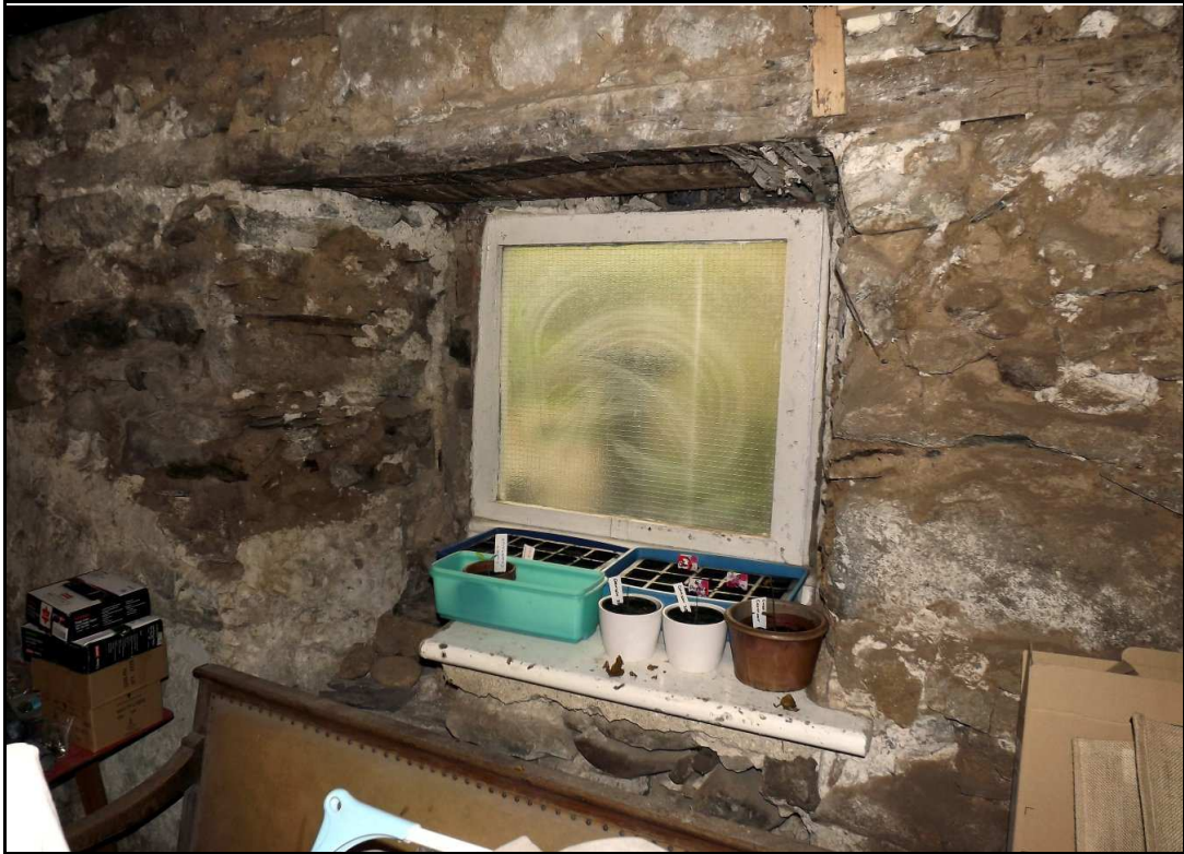
Figure 26, The south-eastern window embrasure in the east range (E). The current sill quite clearly lies upon a later infilling of the original splay.
