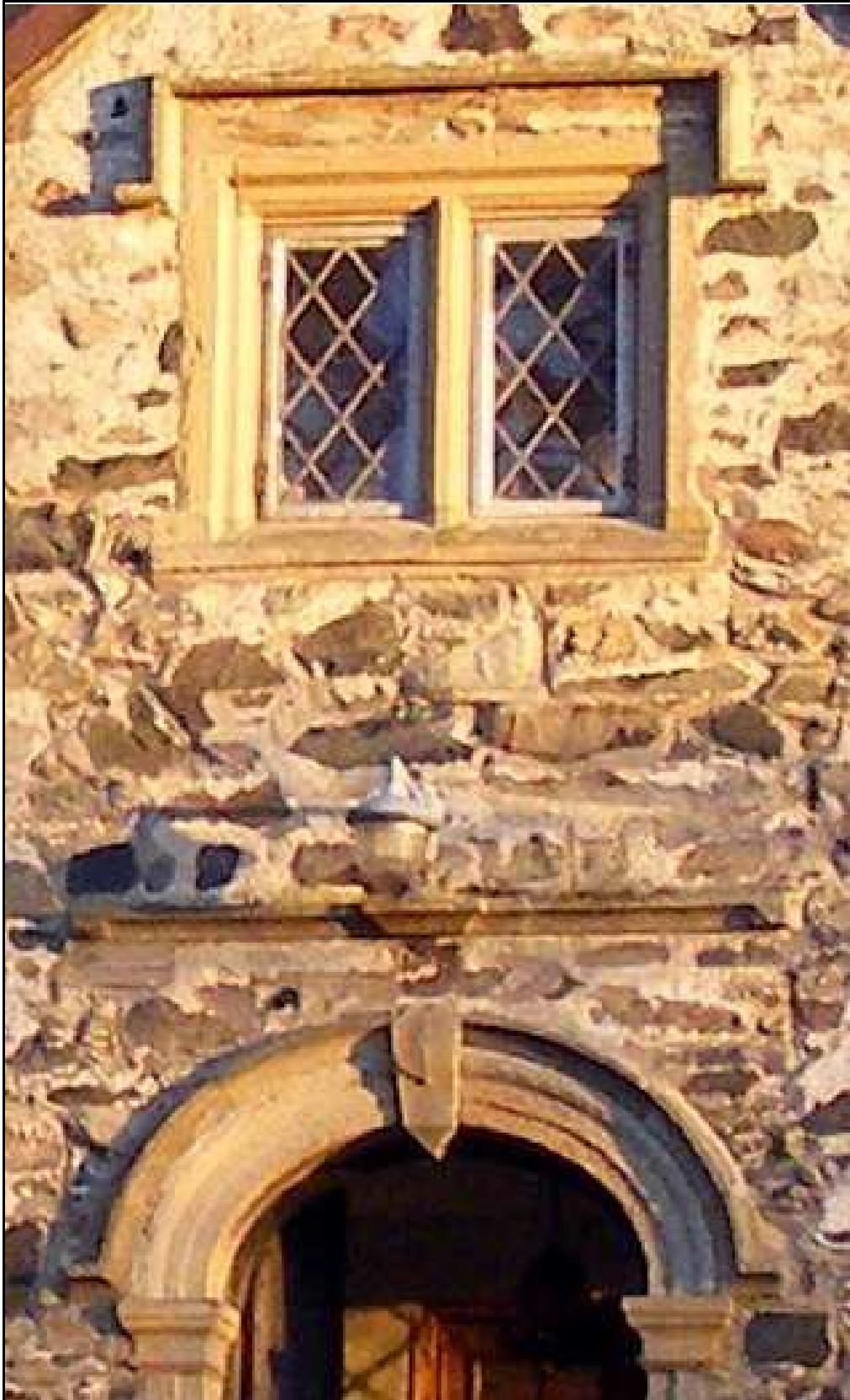
Figure 57 , A close up of the figments around the north facing openings in the porch (P).
