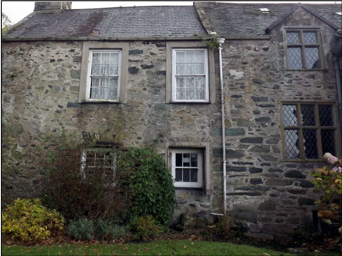
Figure 23 , The converted doorway in the centre still showing the different masonry style at the base where the door has been blocked in.
