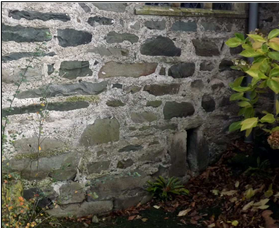
Figure 14 , The eastern basement window. Notice the superior sandstone blocks beneath the light to the east. This would appear to be part of the original building.
