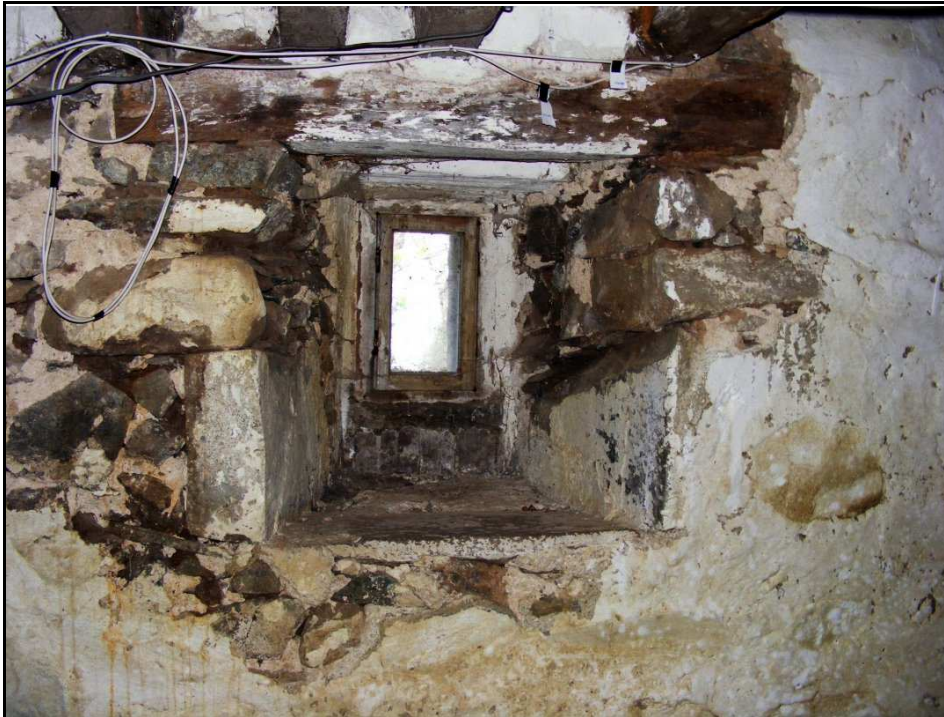
Figure 13 , The remains of the embrasure of the eastern basement (B) window. Notice the two lower quoins and base of the structure and more modern lintel above. Notice the break line between builds running above the two side quoins.
