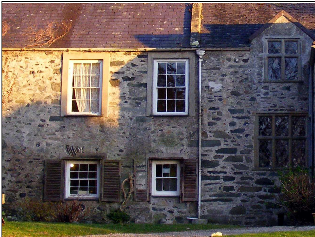
Figure 20 , The east range (E) to the left, divided from the house (H) to the right between the drain pipe and the central windows. Notice the two ground floor voussoirs.
