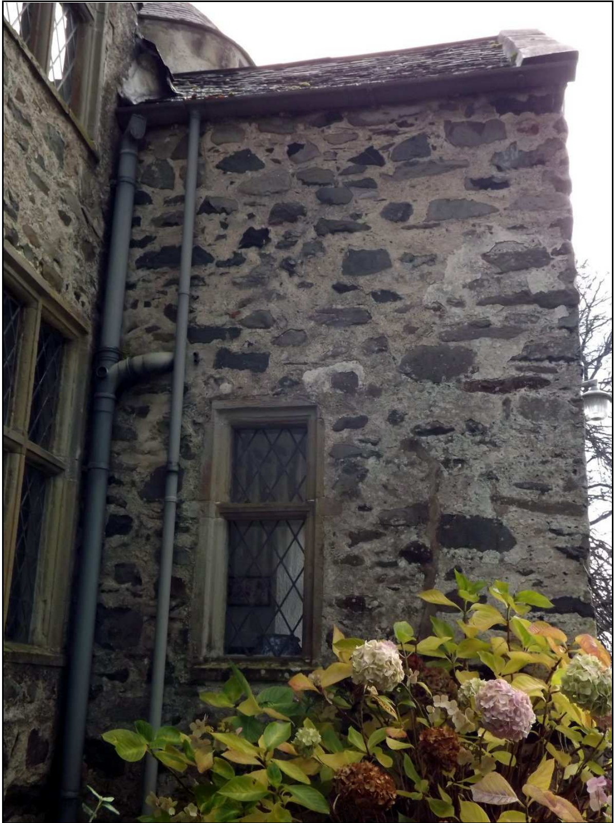
Figure 55 , The east side of the porch (P) showing the fracture line between the replaced corner of the building for the lower three-quarters of its height,
