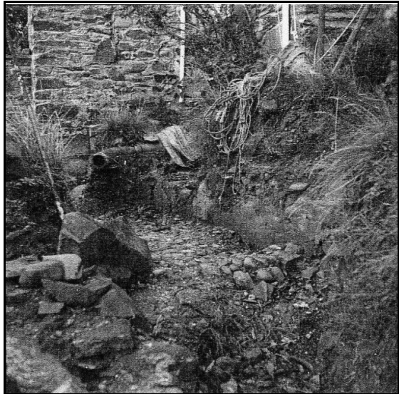
Figure 16 , The 1993 excavation north of the east basement window showing the sandstone blocks to the left by the pipe.
