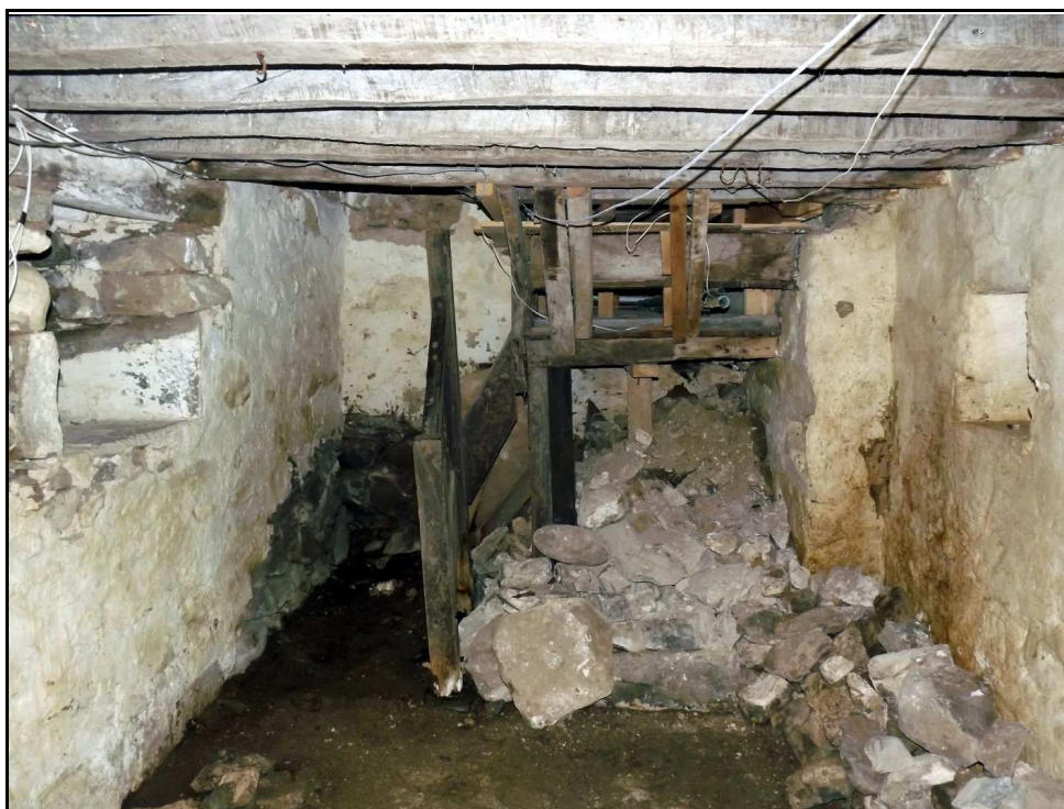
Figure 5 , The eastern portion of the basement (B) with the remains of the old wooden stairs. Notice the wall thickening to the right of the stairs. The beams of the 1970's floor make up the current ceiling of the cellar.
