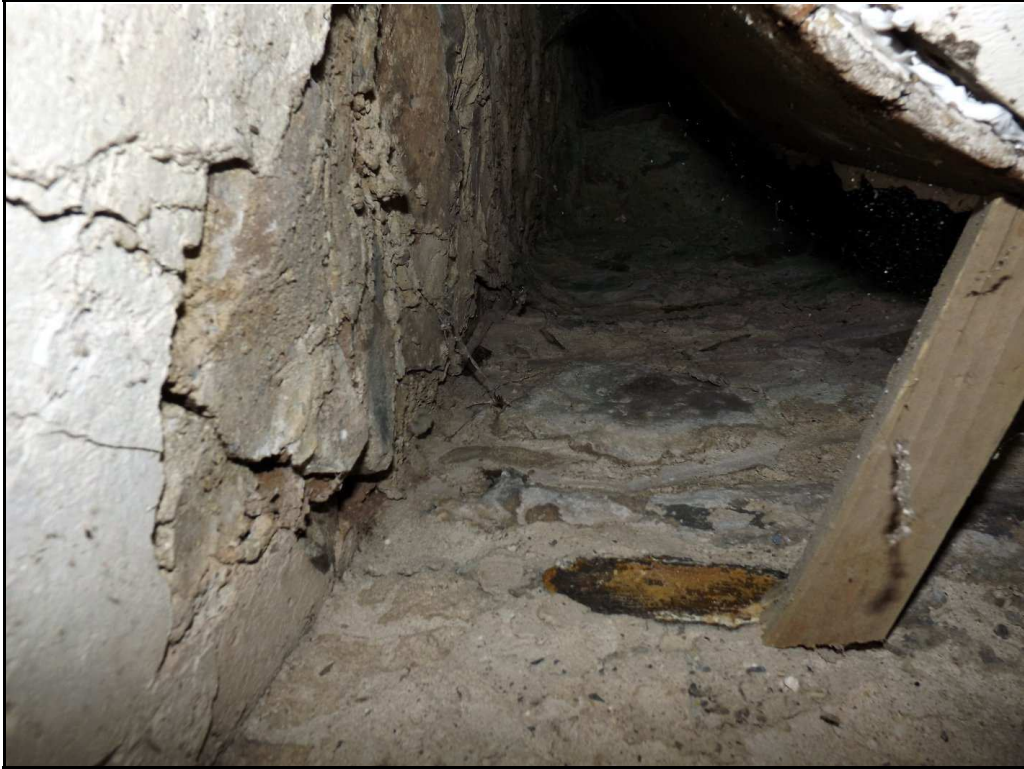
Figure 39 , The blocking wall in the passageway in the south-west corner of the house (H) to the left. The tower (T) wall is to the bottom right and the back of the fitted cupboard to the top right.
