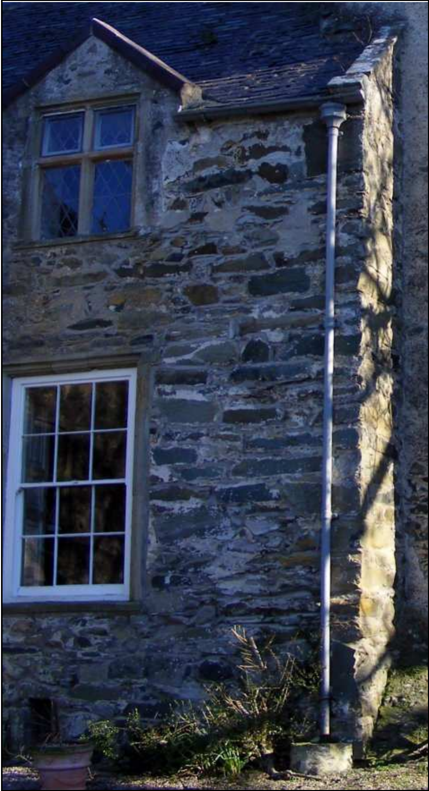
Figure 37 , The north-western corner of the house (H), showing its regular build and few quoins.
