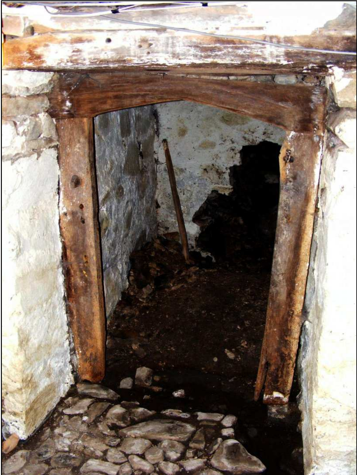
Figure 10 , The doorway from the basement (B) into the basement of the porch (P). This has a sixteenth century 'feel' to it, the arched header, if not the jambs could be this old. Note the angle of the right hand jamb and the two hinge pivots, the lower one missing. No door could have hung here with the jamb at its current angle. Most likely the whole thing was reset in the 1970's when the floor above was laid.
