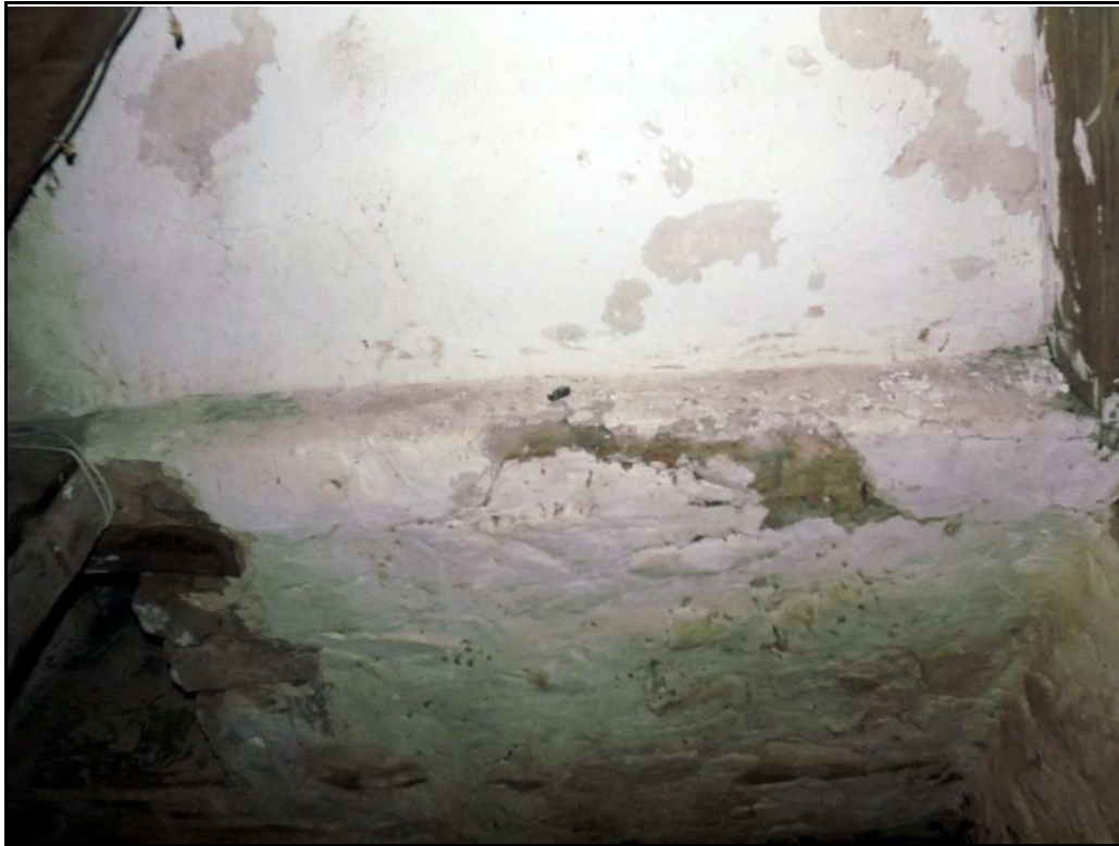
Figure 7 , The floor offset in the basement (B) seen from the ground floor level of the house in the old stair well.
