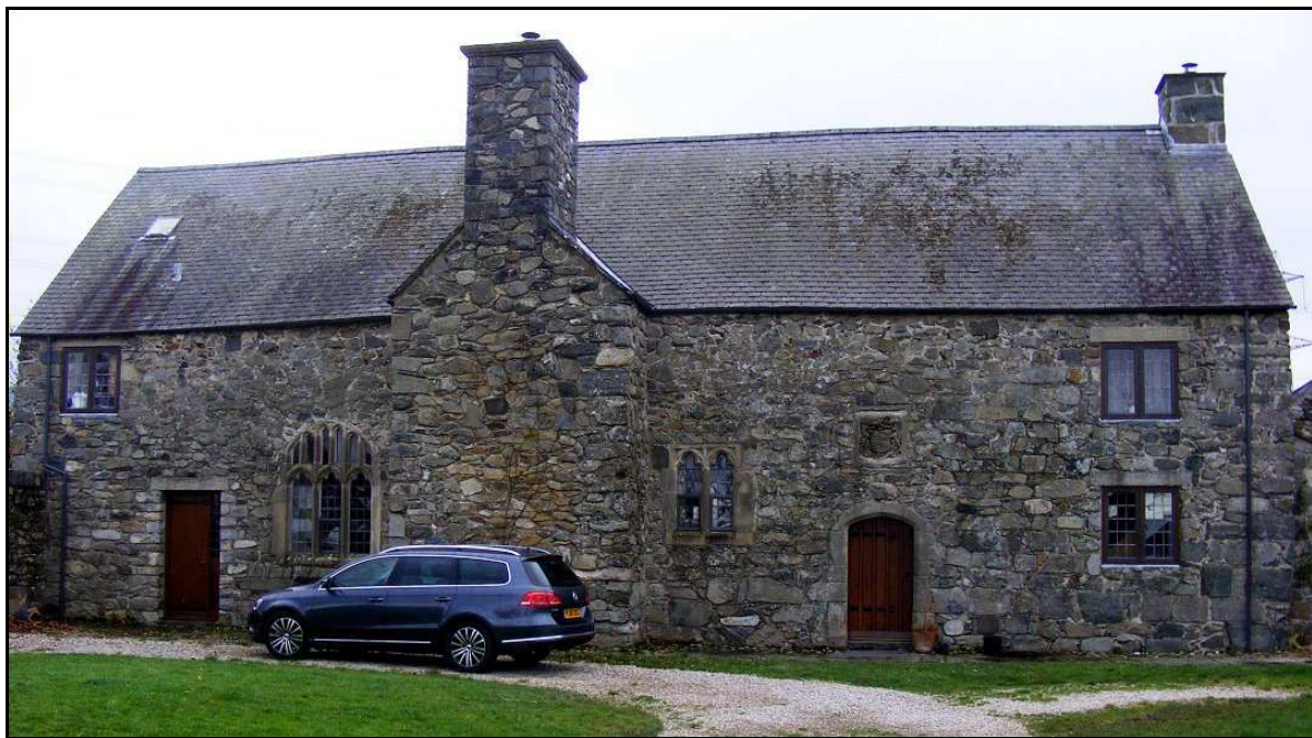
Figure 83 , Cochwillan from the north showing the multiple building phases and inserted fenestration.
