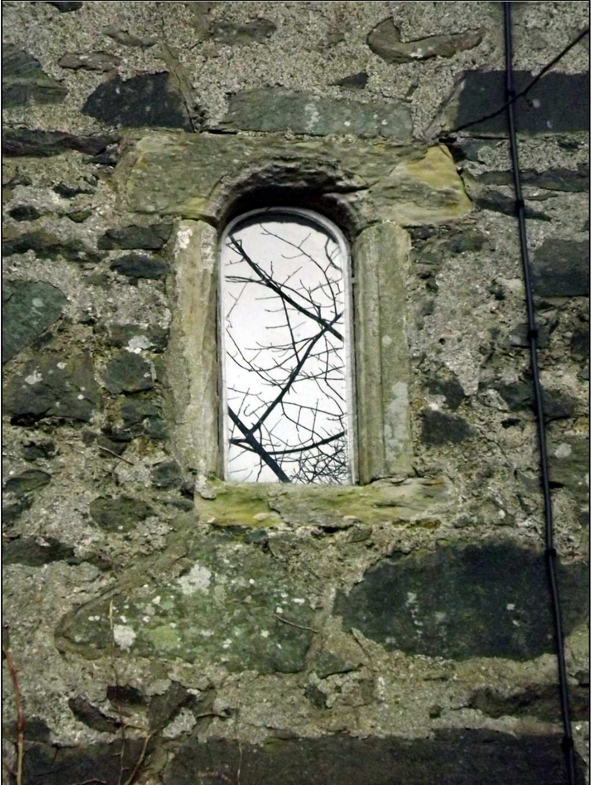
Figure 50 , The arched window in the west wall of the upper storey of the south range (S). Note the decoration.
