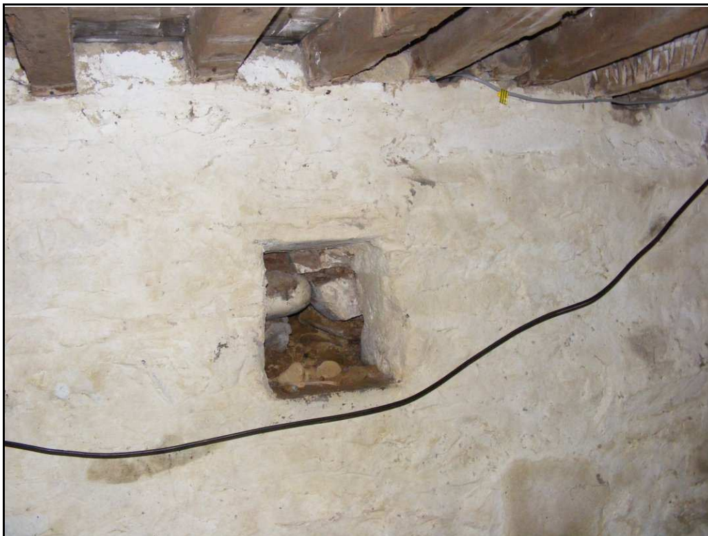
Figure 8 , The westernmost niche in the cellar wall in the basement (B) showing the rubble filled packing in the adjacent chamber.
