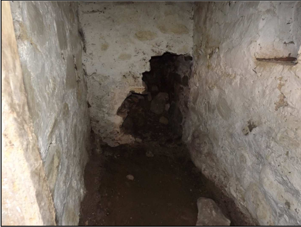
Figure 58 , The breach in the north wall of the porch basement. Notice how both side walls make a butt joint against the older north wall. The niche is just visible top right.
