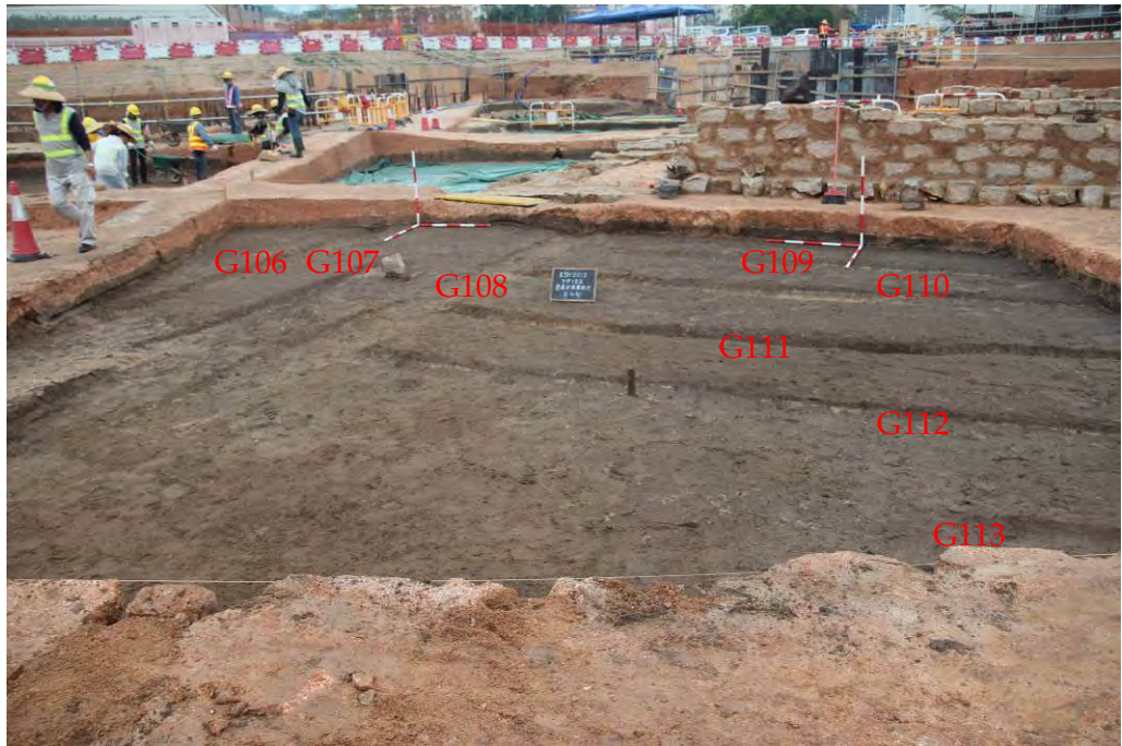
Figure B4p Ditches G106 to G113 unearthed in TP122 (South to North)
