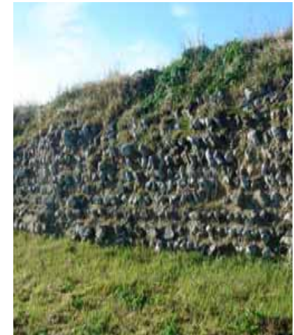
Roman wall on eastern facade - identifies extent of main element of Roman Fort
