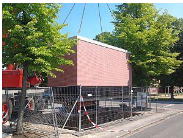
Die „Point of Presence“ - Station in Hetzerath
