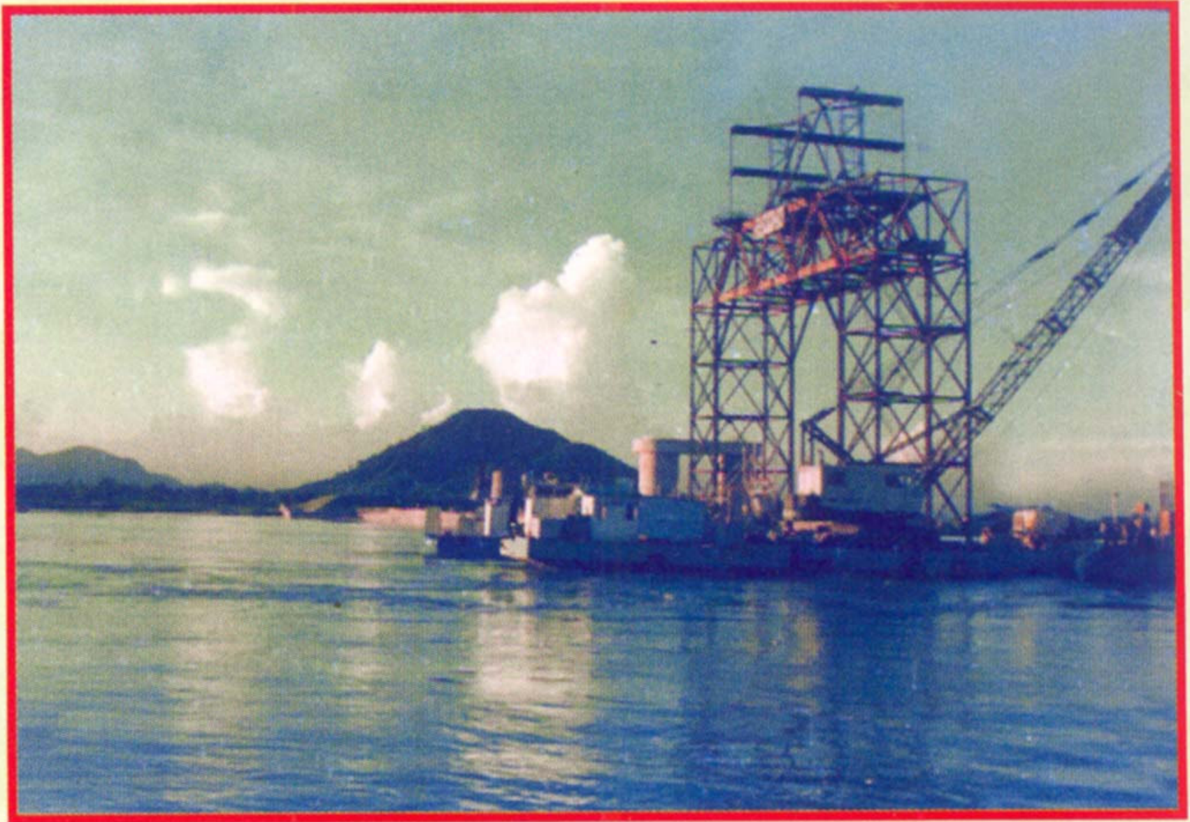
Gantry on barge for transporting caisson on river and placing it in position
