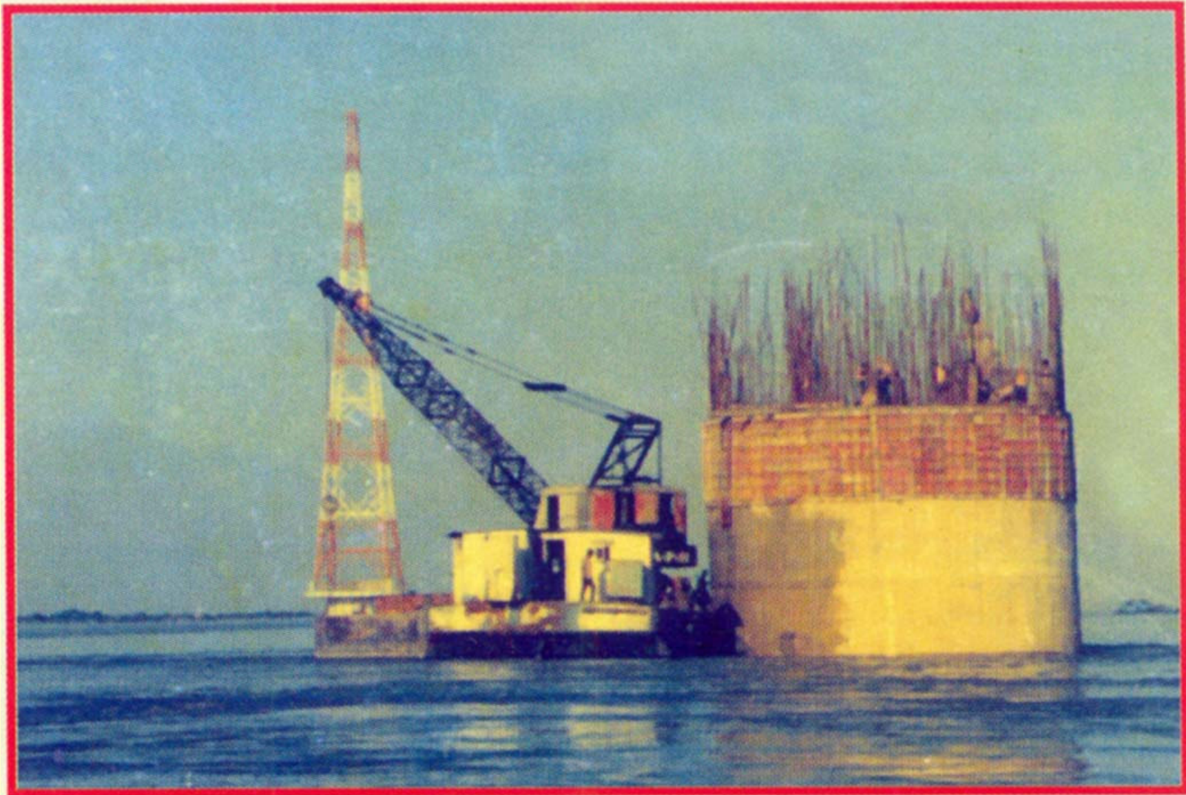
Tilted pier no.-13
