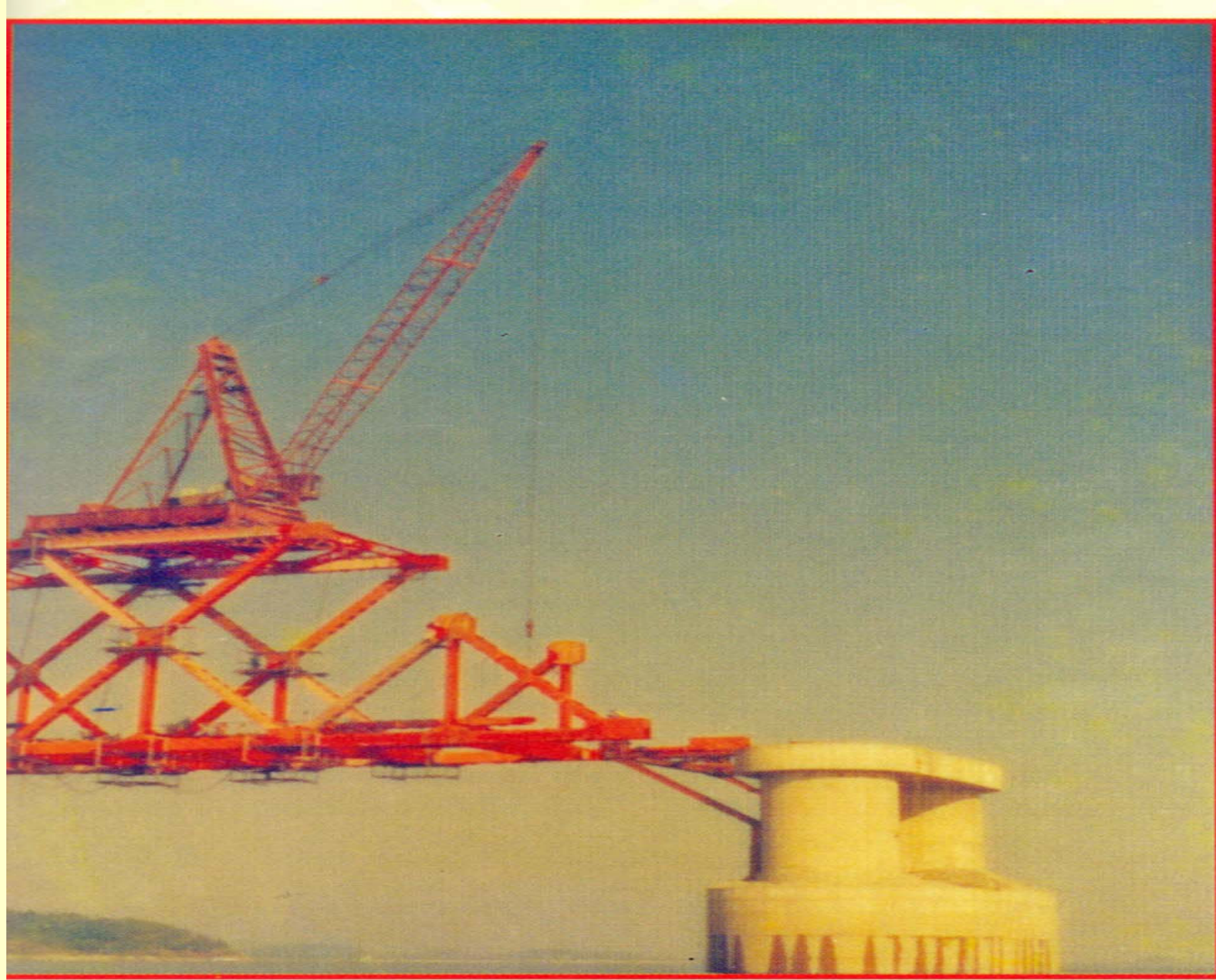
Full length cantilever span being held by temporary Receiving bracket to reach pier cap
