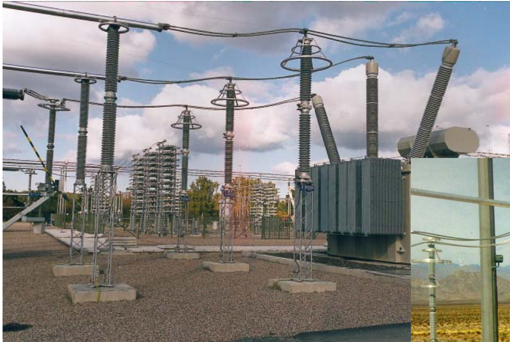
SwePol Link, Shunt reactor bay at Slupsk
