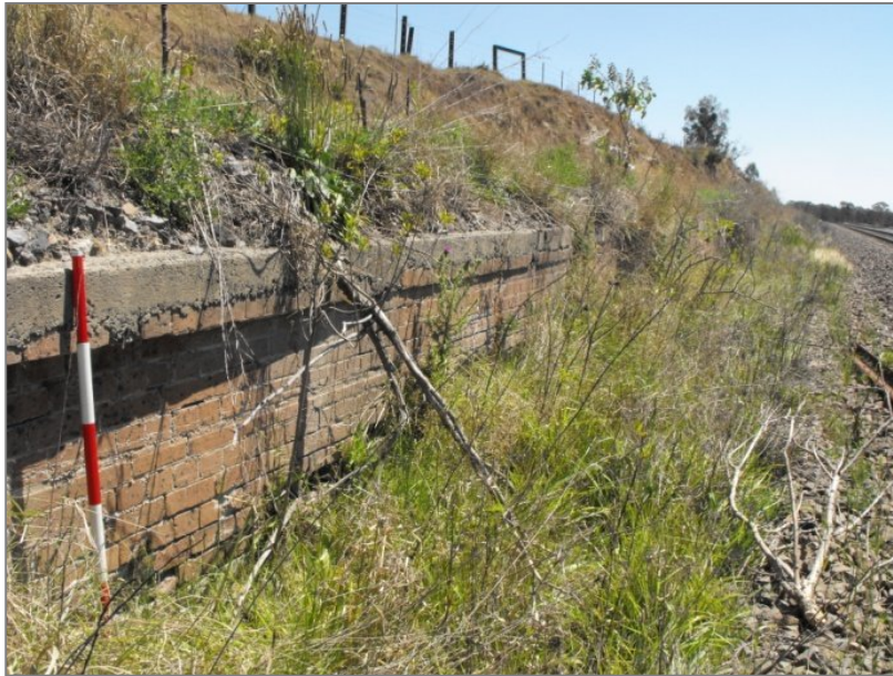
Figure 2.8 View of brick platform face of the former Farley Railway Station looking downline. Note brickwork laid in English Bond. Photograph by Sue Singleton, November 2009.
