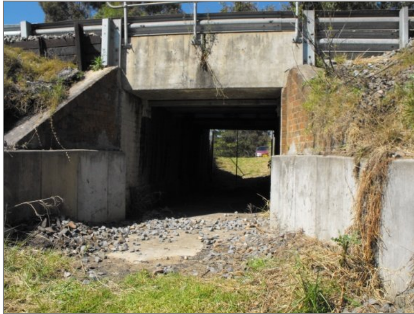
Figure 2.9 View of box culvert used for stock crossing. Thought to have been constructed circa 1860. Photograph by Sue Singleton.
