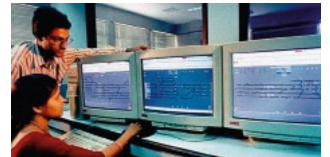
Signalling Control Room, Traffic Control System
