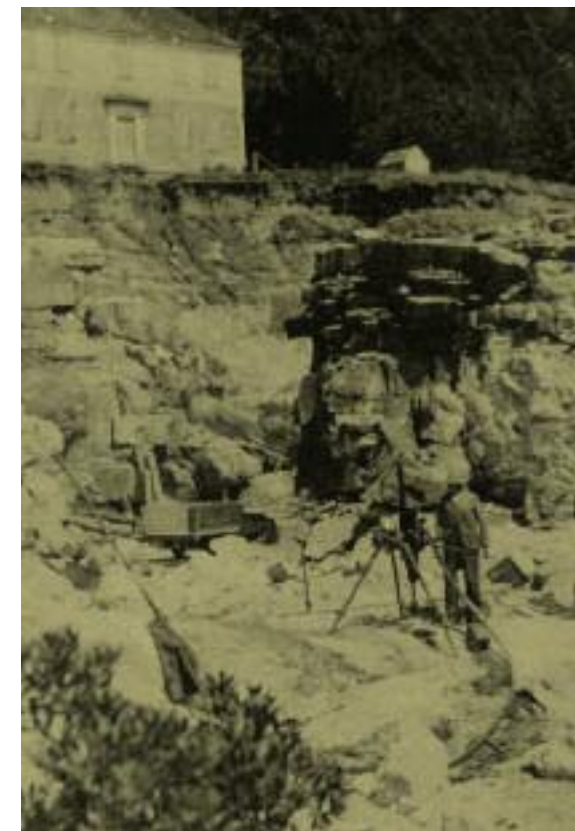
Drilling into the quarry floor in preparation for blasting. The Gillette Quarry, Haddam Neck, c. 1890s. Started by M. P. Gillette in 1896, the quarry was leased by an affiliate of Tiffany & Co. from 1905 to 1909 to mine for gemstones. photo: Charles R. Harte
