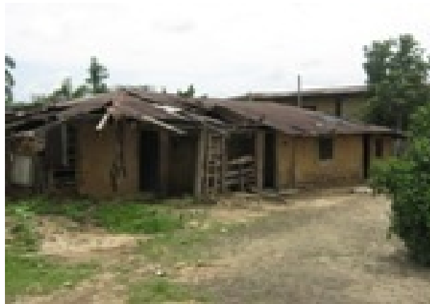
Plate 5. Mud house ravaged by strong winds in Ndoni (RULIN field survey, 2010)
