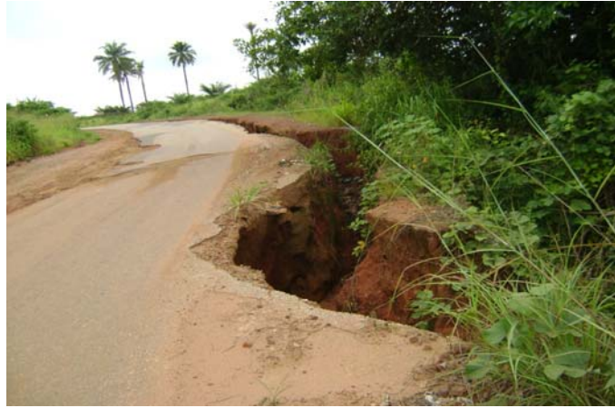
Figure 11 Developing gully along the road to Akanu-Ukwu Ohafia, in Abia State
