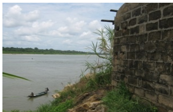
Plate 3. A building under construction abandoned by the owner due to river bank erosion (RULIN field survey, 2010)
