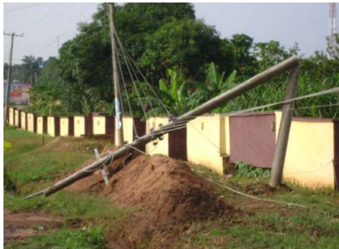
Figure 10 Wind damage to electric poles at Umudike, Abia State
