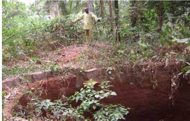
Figure 22 Flood reception pit at Isuofia, Anambra State prevents flooding of roads
