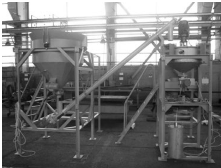
Figure 3. Overall view of cementation plant
