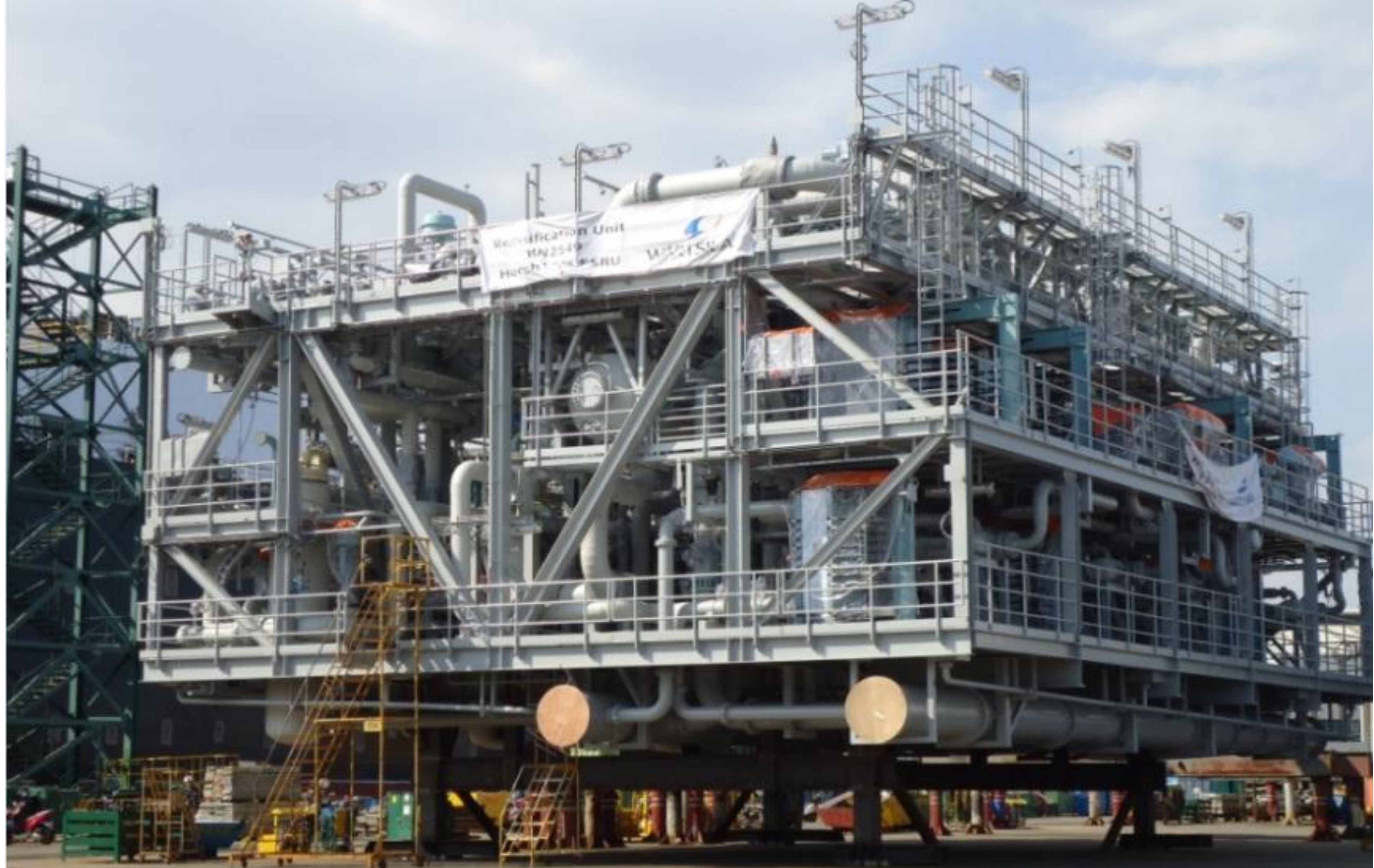
The regasification unit, mounted on the FSRU, tested and certified by the end of June, 2013
