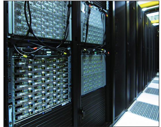
SM15000 servers and Freedom Fabric Storage FS 5084-L units deployed in the Verizon Terremark data center
