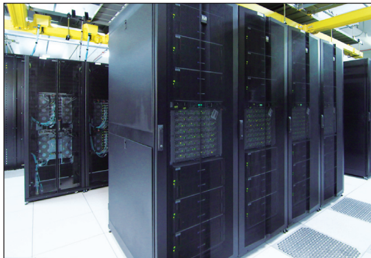
The Verizon Terremark data center
