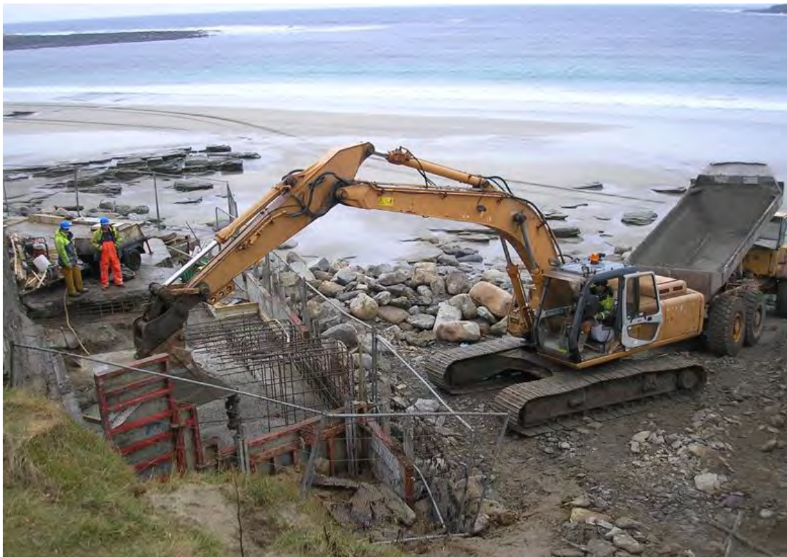
Works to extend the toe of the sea wall at Skara Brae
