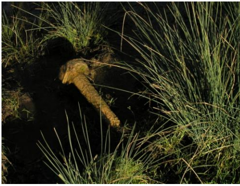
Remains of the pipe ducting water from Knightswood spring in Birdcombe valley to Nailsea ST 475 717
