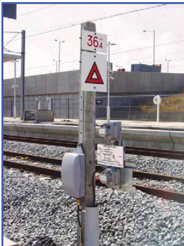
Emergency Replacement Switch Location
