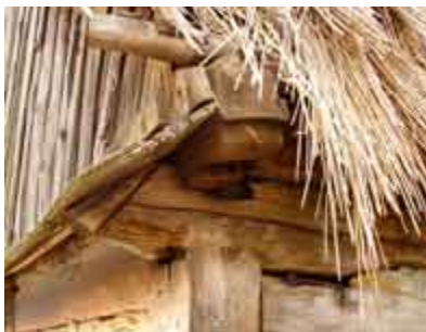
Gable extended beyond side wall's face in a building
